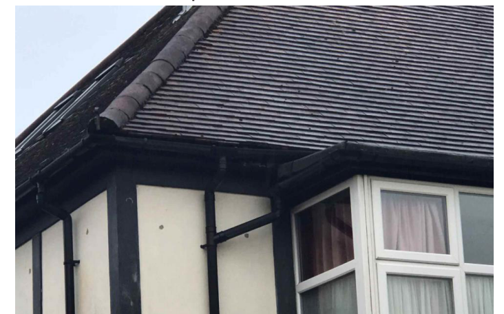
Uneven roof tiles to eaves be re-laid or replaced
