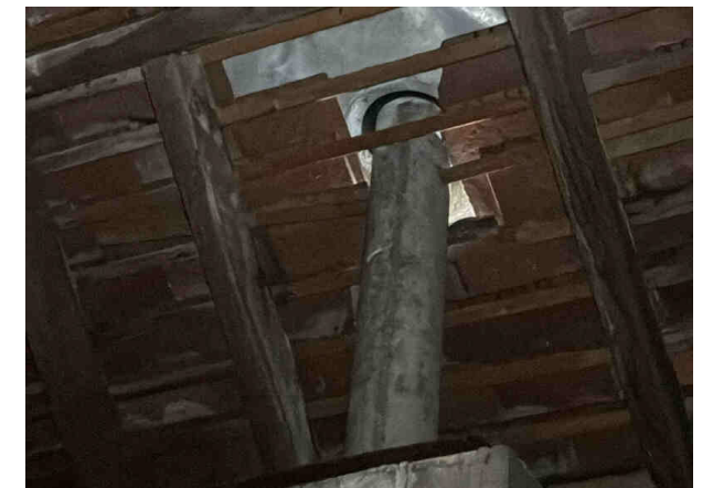
Asbestos found in existing chimney flue pipe.
