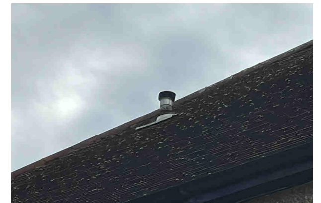
Presumed Asbestos flue cowl.
