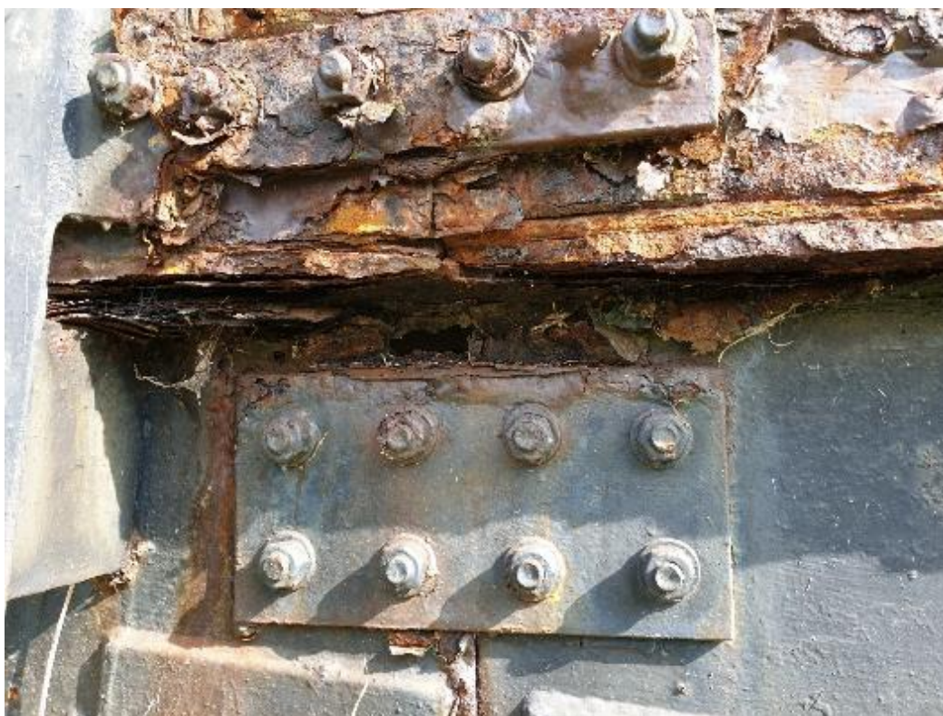
Typical corrosion and section loss at connection to steel beam
