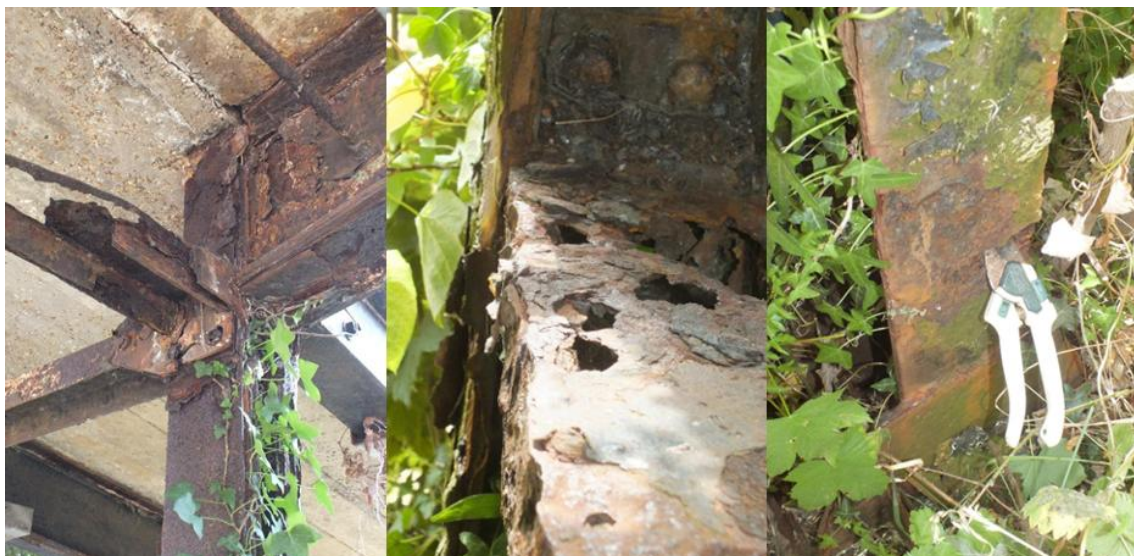
Deterioration of the northwest ramp
