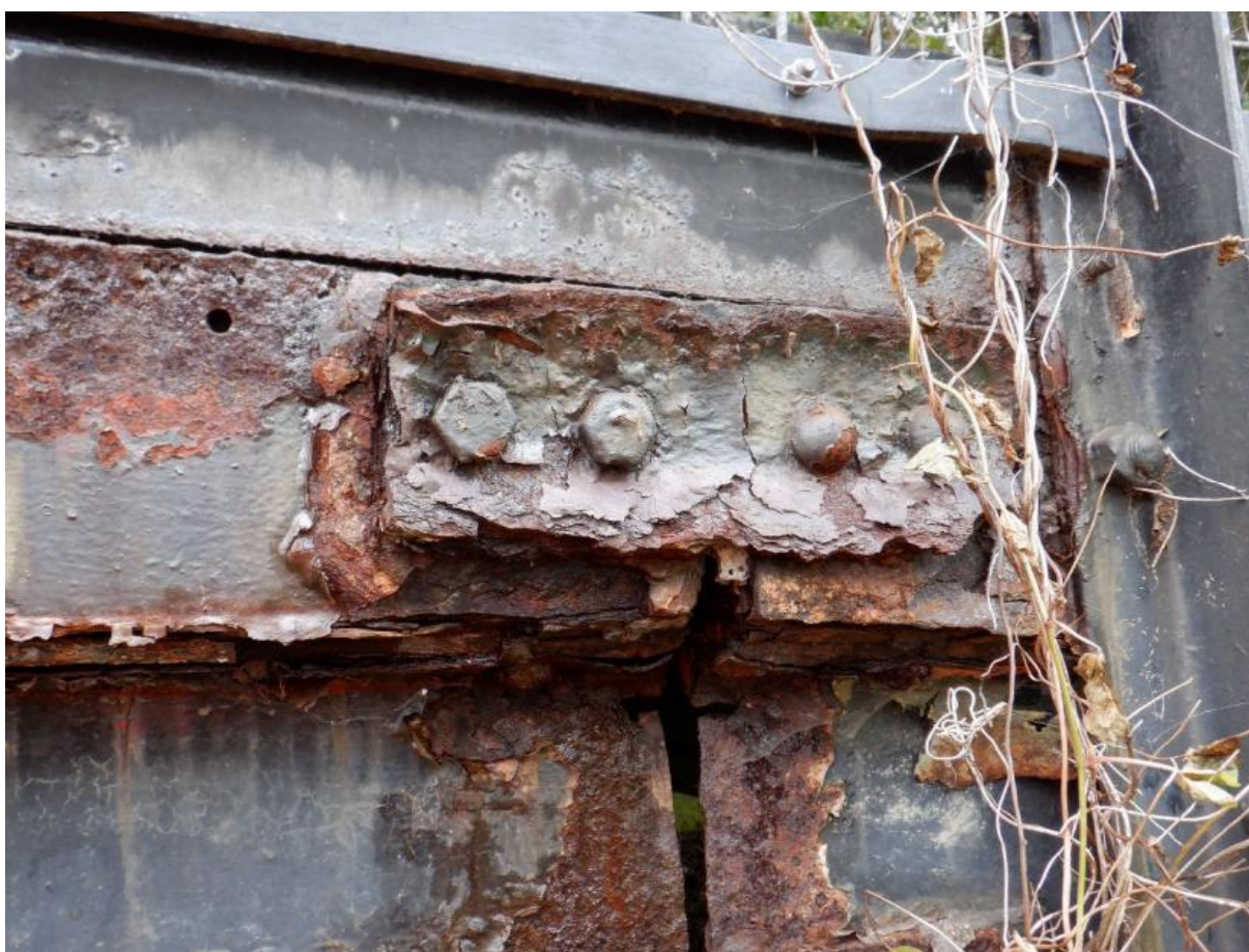
Typical delamination and knife edging to steel beam
