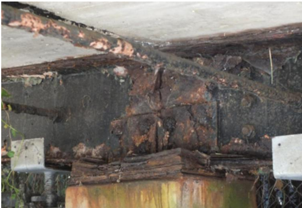
Typical corrosion at support locations.
