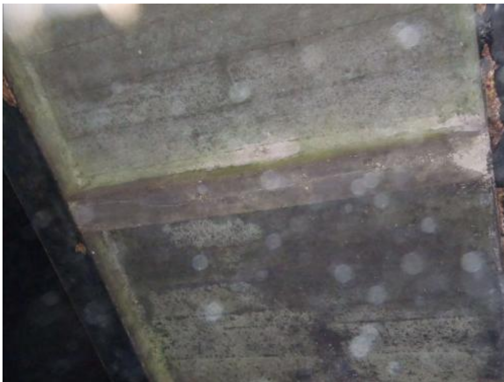
Main span – typical view full length crack to concrete
