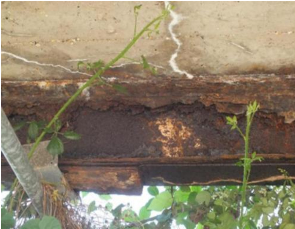
Typical corrosion underneath the ramps
