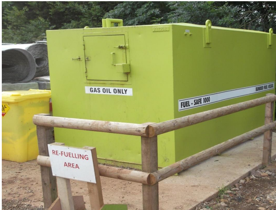
Figure 10 - Example of a protected refuelling area on handstand with spill kit
