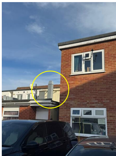
Figure 7 – Extraction unit from restaurant to the rear
