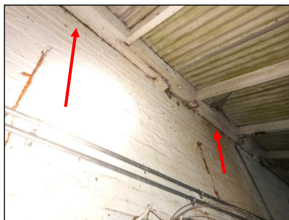
Photo 8 Room 62, southern elevation. Gaps between timbers and brickwork
