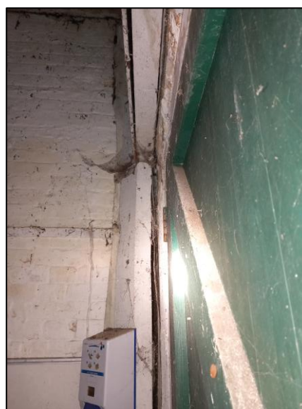
Photo 10 Room 62 – gaps around door at western end
