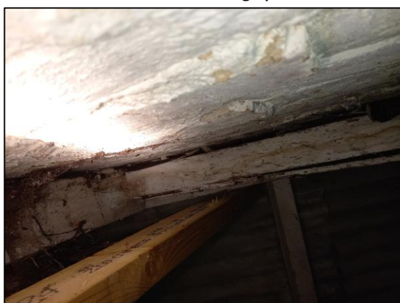
Photo 11 Room 62 – gaps between boarding and wall
