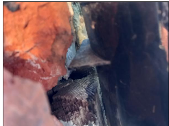
Photo 16 North-eastern corner of Potting Shed Gap between timbers and brickwork.
