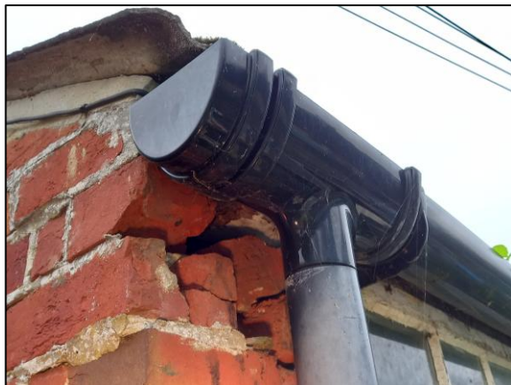
Photo 15 North-eastern corner of Potting Shed, crumbled brickwork
