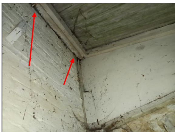
Photo 7 Room 62, south-western corner. Gaps between timber and brickwork.
