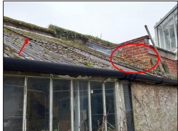
Photo 14 Lifted corrugated roof materials indicated with arrow, area of crumbled brickwork in circle.
