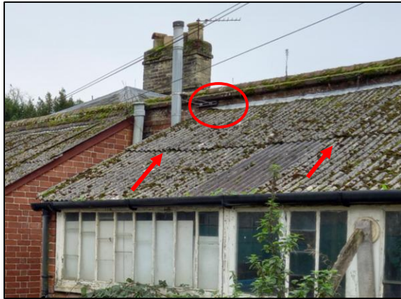
Photo 13 Lifted flashing indicated with circle, gaps in corrugated roofing material indicated with arrows
