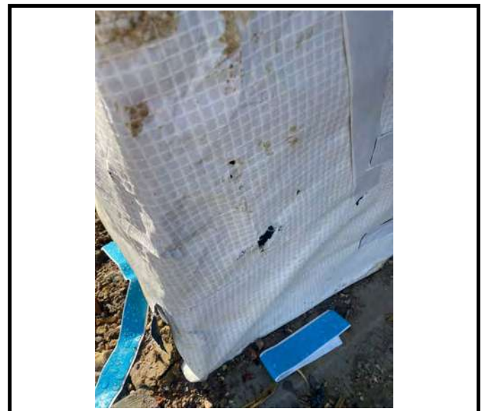
Holes and defects were incorrectly sealed with double sided butyl tape.
