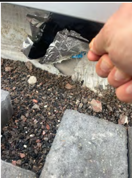
Several areas of damage identified.
