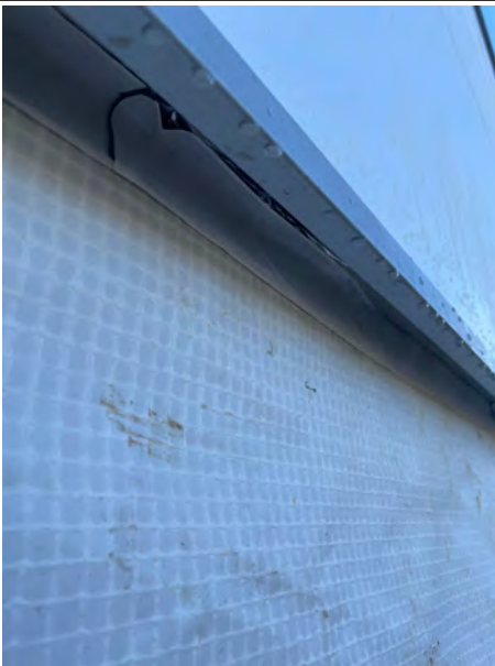
Insufficient installation to the perimeter due to the dual taped system not being correctly implemented.
