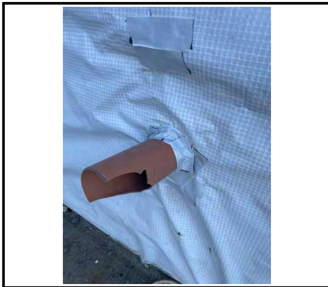
A pipe penetration incorrectly sealed with double sided butyl tape.
