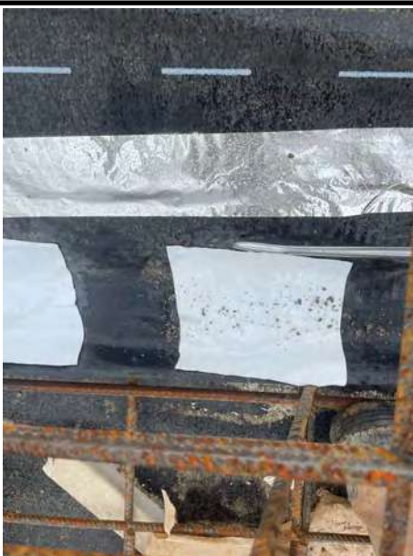
Additional photo of a mechanical stress point test being carried out to a sealed to a repair.
