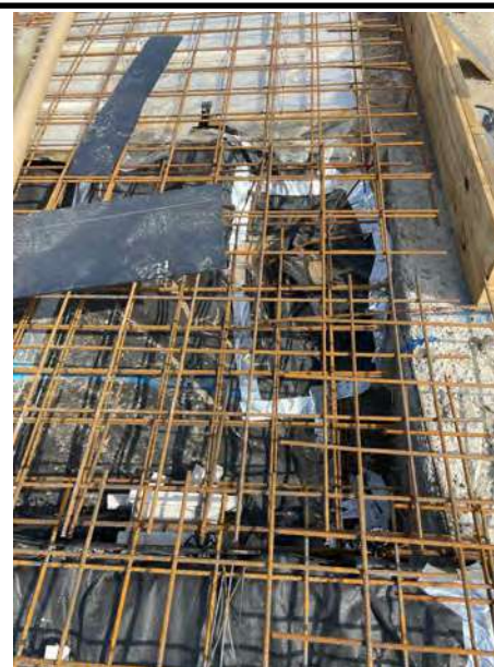
Photograph of outstanding area that requires remediation, still will need to be removed prior to repair.
