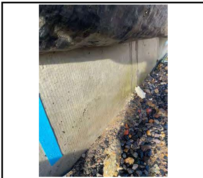
Holes and defects incorrectly sealed with double sided butyl tape.
