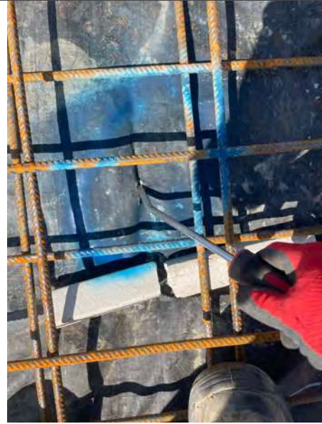
Additional image of identified fault
