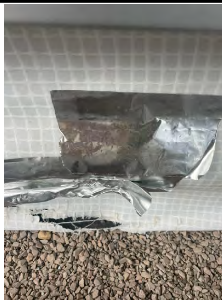
The tapes have not correctly adhered to the membrane.
