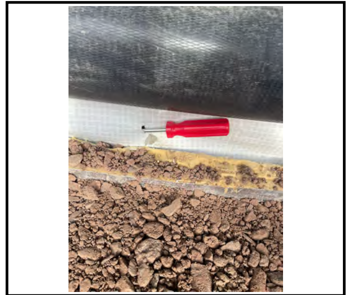
A puncture identified in the membrane.
