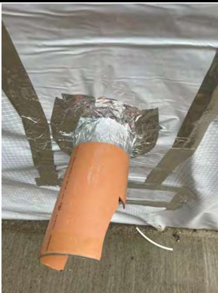
Insufficient installation to the perimeter due to pipe penetrations sealed incorrectly.
