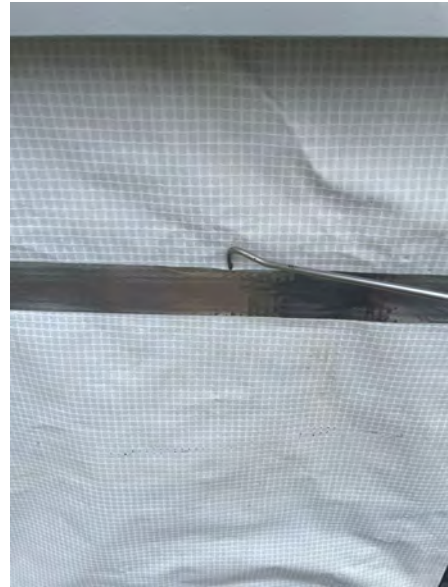
A mechanical point stress test being conducted upon a taped lap joint.
