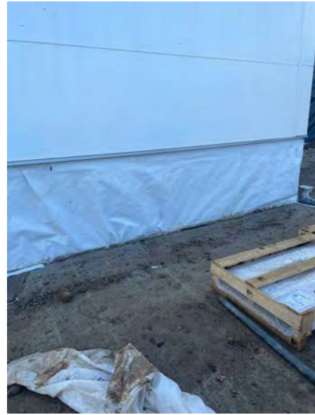
Insufficient installation to the perimeter due to the dual taped system not being correctly implemented.
