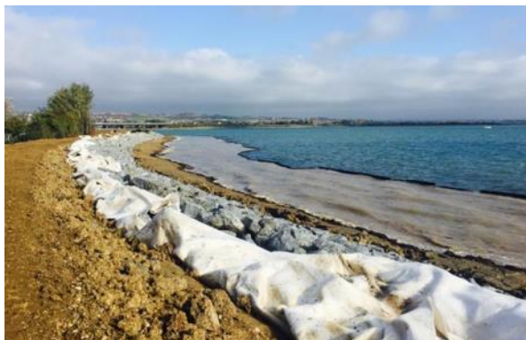
Figure 4.1: Silt curtain in good working condition.
