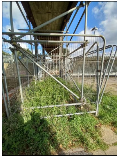
Photo 18 Vegetation beneath ramp south of station.
