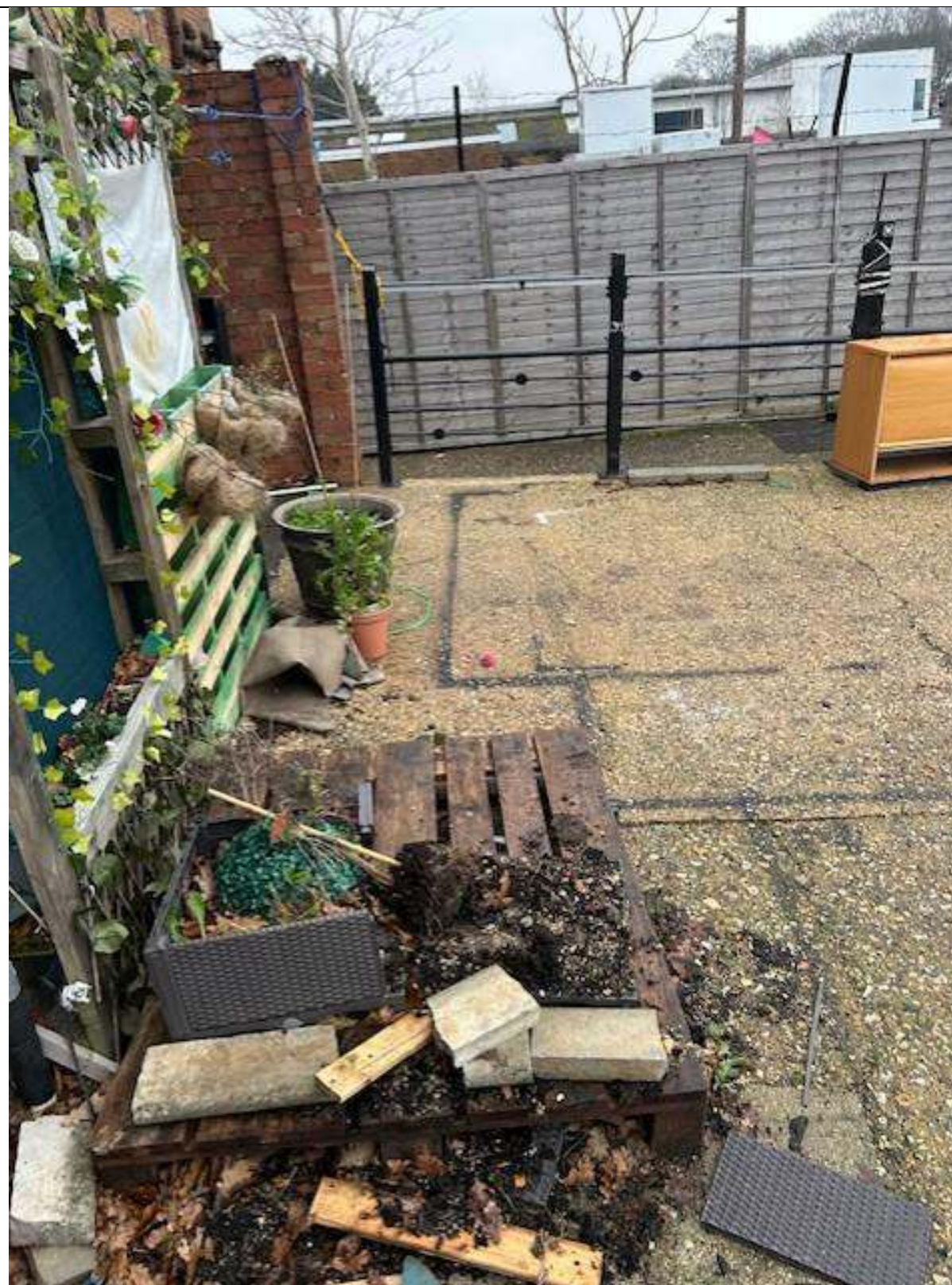
Photo 5: A small pile of rubbish noted outside the building on top of hardstanding ground.
