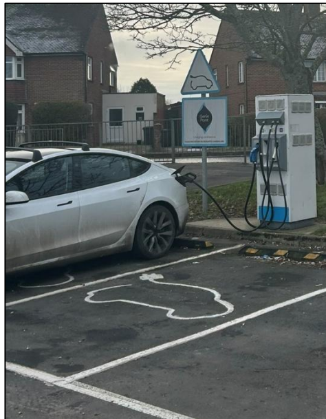
Photograph 17: EV charging spaces
