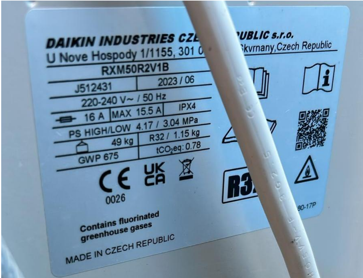
Photo 5: Daikin Spec plate (unit 4)
