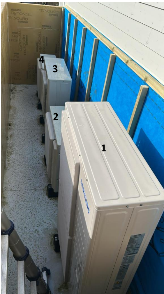
Photo 1: 4 units in enclosure (blue lining to house façade)
