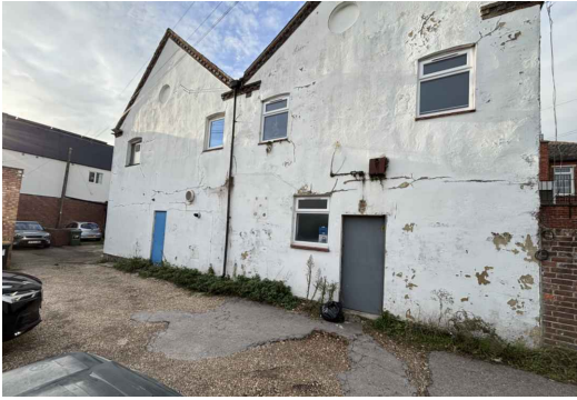
Existing rear elevation Walls are pale painted render in poor condition.
