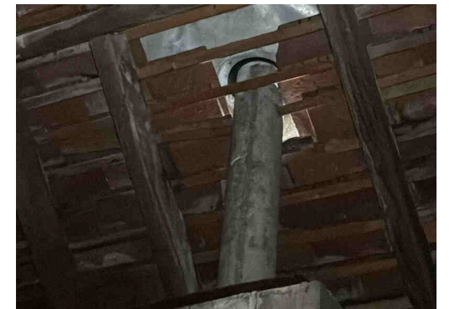
Asbestos found in existing chimney flue pipe.
