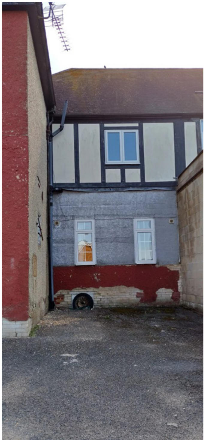
Rear Elevation ~No.9 -render is in poor condition
