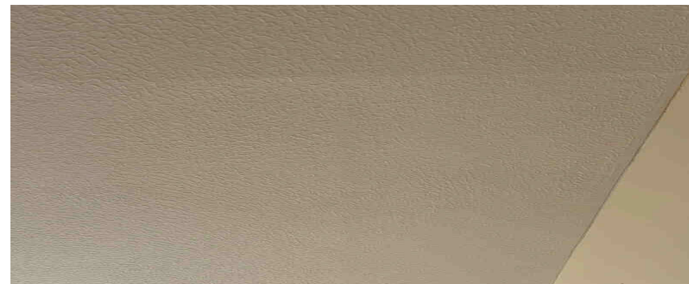
Textured ceiling- strongly presumed Chrysotile
