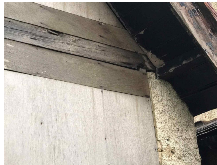
Existing timber soffit , verge and eaves to existing garage needs to be replaced and cracks in facade made good.
