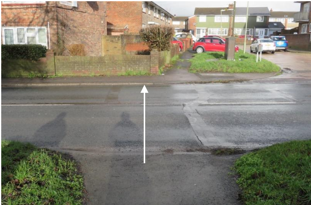
Photo 4: Proposed tactile paving will be abutting a full height kerbline and a transition kerb (head of the arrow)
