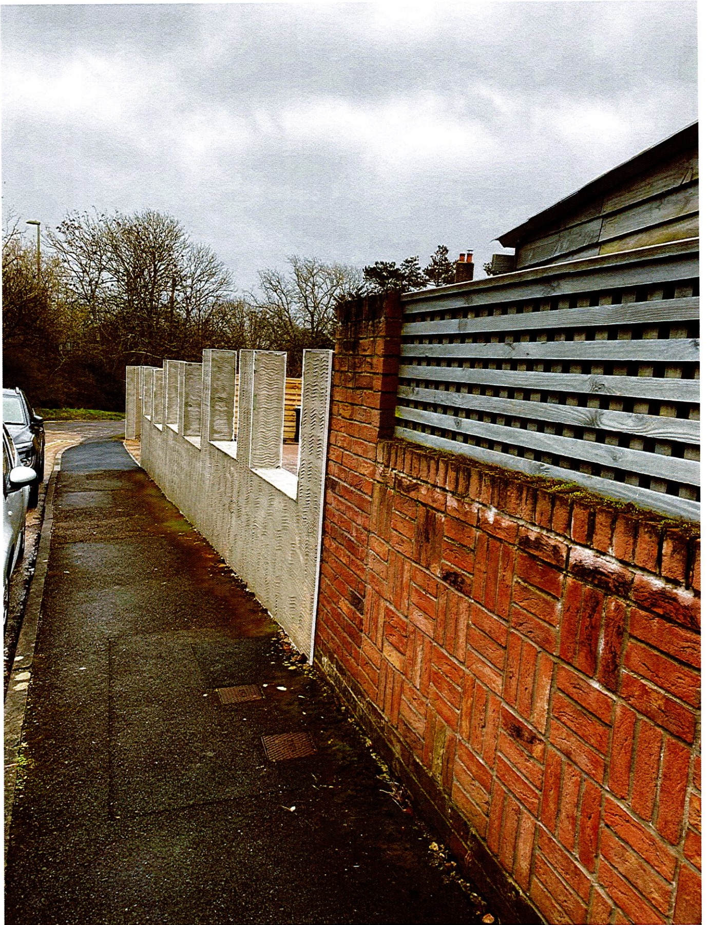
Wall to the right 28 HULBERT ROAD.
