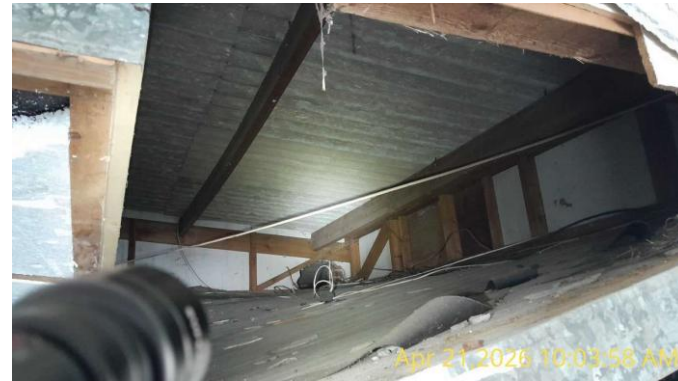
Showing another look at the internal area, with a partially collapsed roof.
