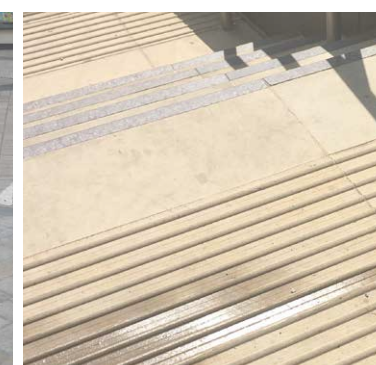
Accessibility - suitable tactile corduroy paving
