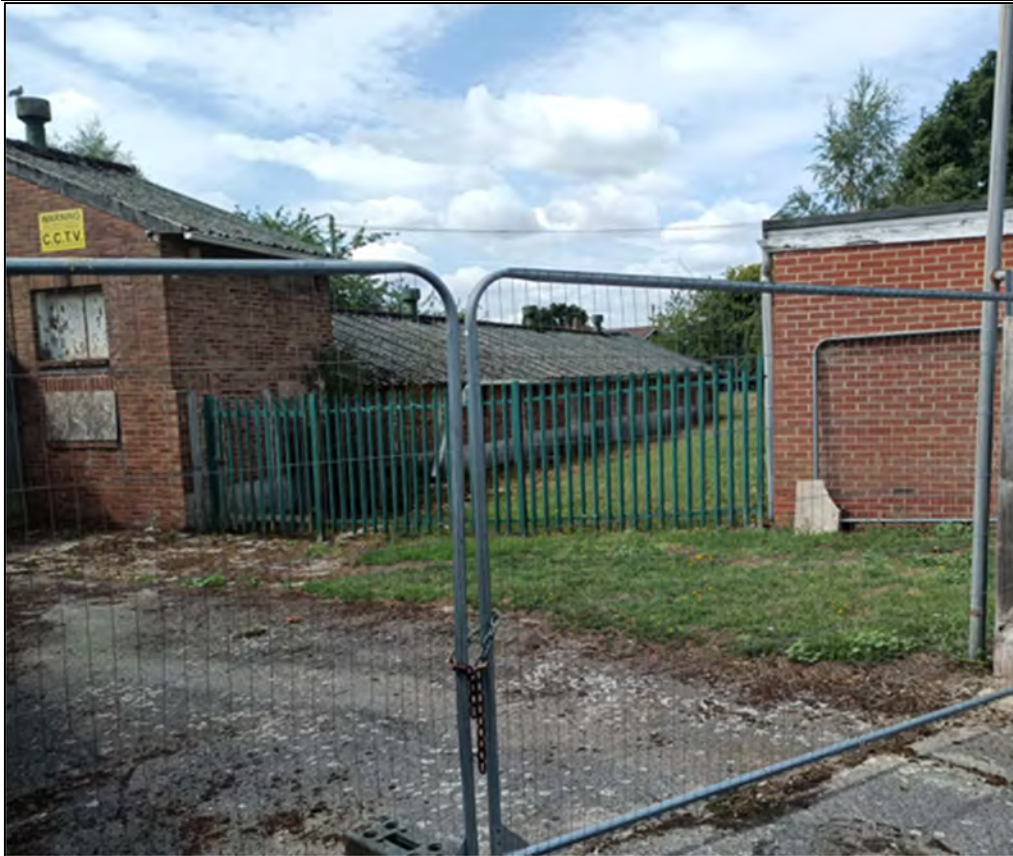
Photo 7: Potential Asbestos containing materials on dilapidated farm buildings.
