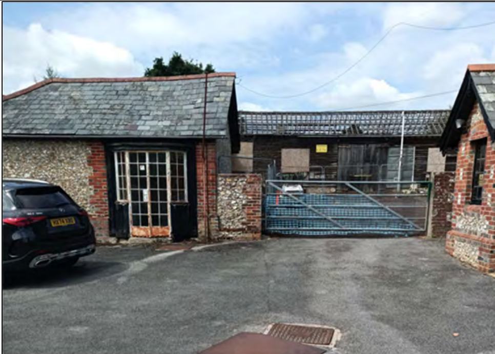
Photo 3: Dilapidated Farm buildings onsite near the southern boundary.
