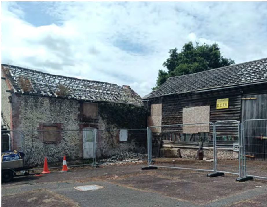
Photo 2: Dilapidated Farm buildings onsite near the southern boundary.
