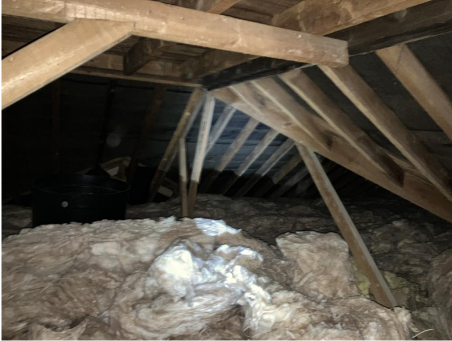
Photograph 17 – Junction of original construction and extension in roof void. Right hand timbers appear to be replacement roof to the original layout. The flat roof to the left is a reconfiguration of the roof for the extension.
