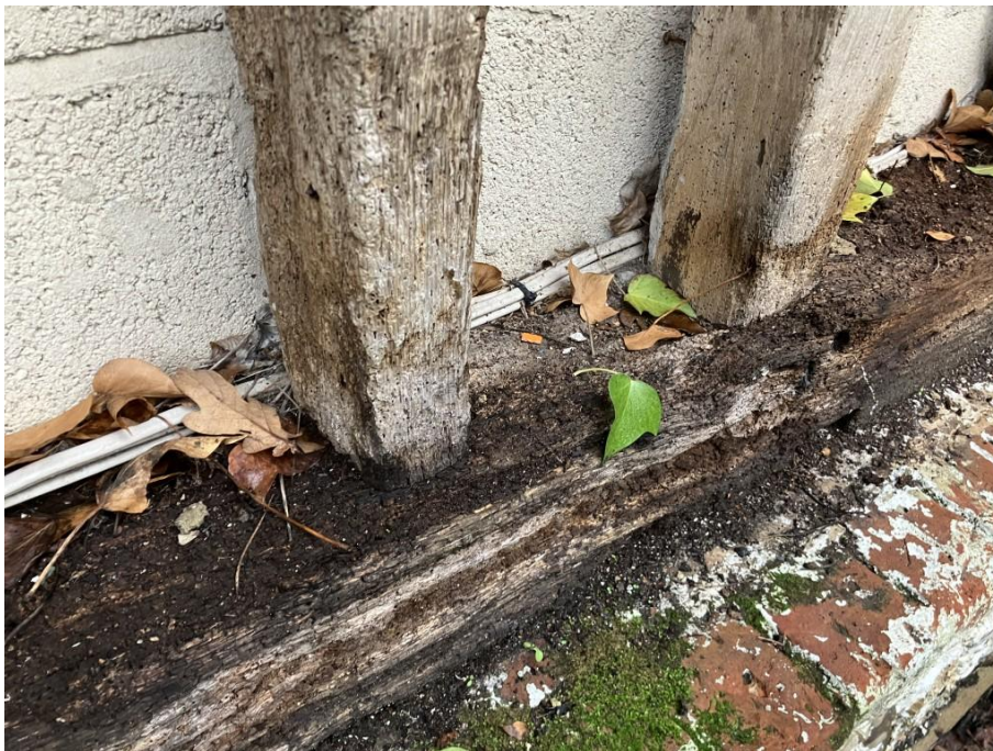
Photograph 28 – Timber decay in mortice and tenon joists at sole plate of east elevation.
