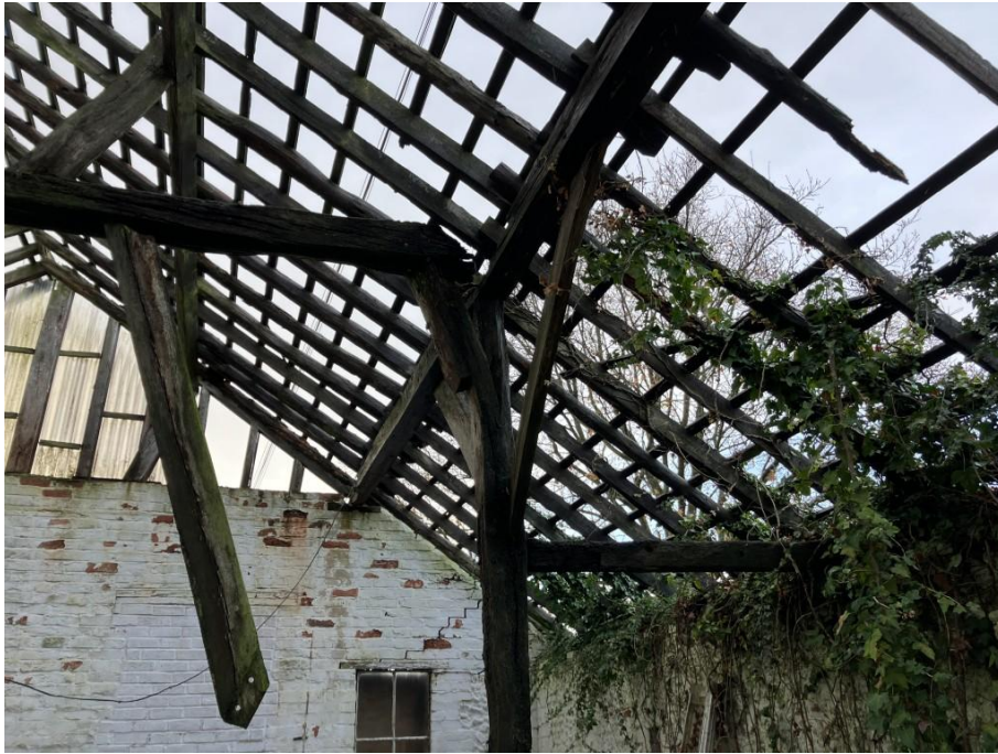
Photograph 33 – Severe damage to timber frame including failed diagonal brace, and severely degraded and split timber post.
