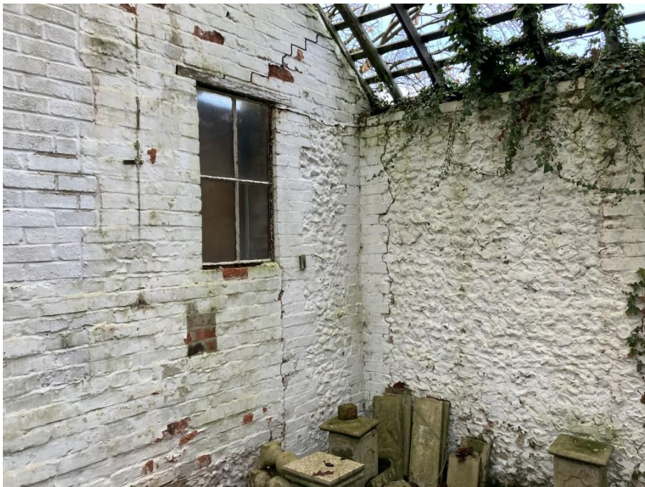
Photograph 30 – Cracking of brickwork infill wall to south elevation (left hand side) and minor separation of brick and flint of original wall to right hand side.
