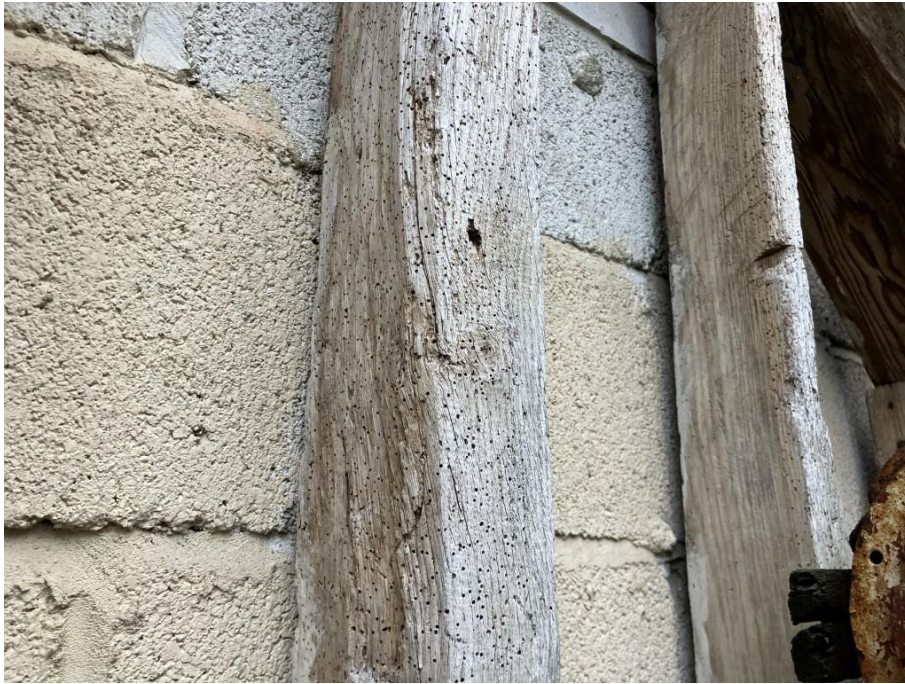
Photograph 31 – Insect infestation of timber studs at north elevation.
