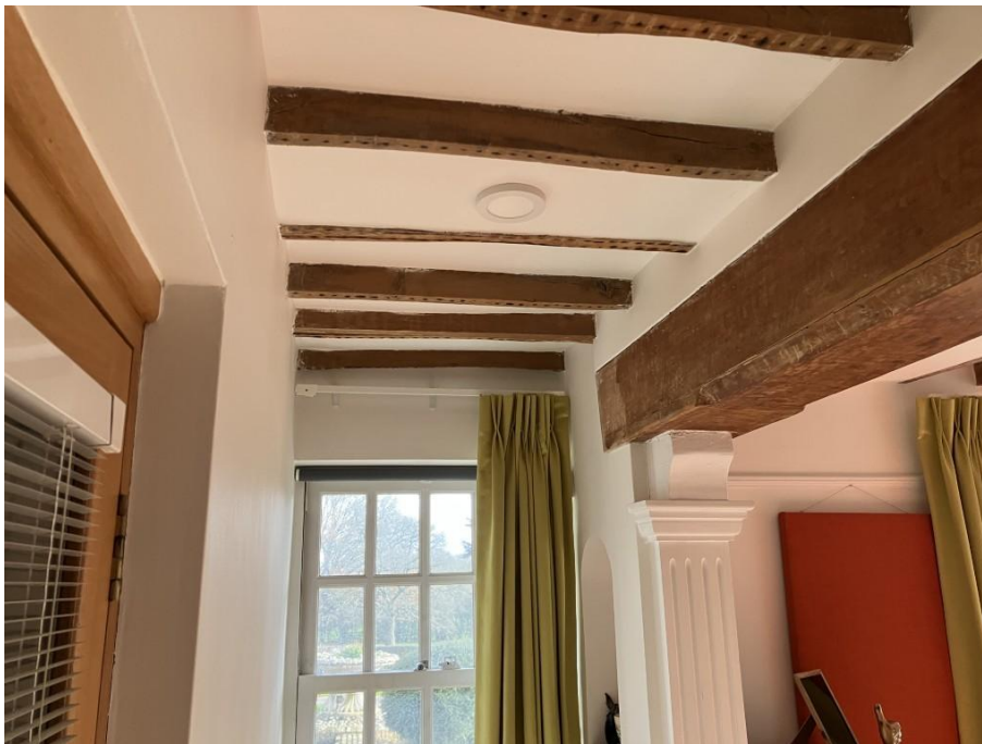
Photograph 10 – Exposed ceiling joists in original hallway. Wall to right hand side removed and supporting beam assumed to have been installed and boxed with cosmetic timber.
