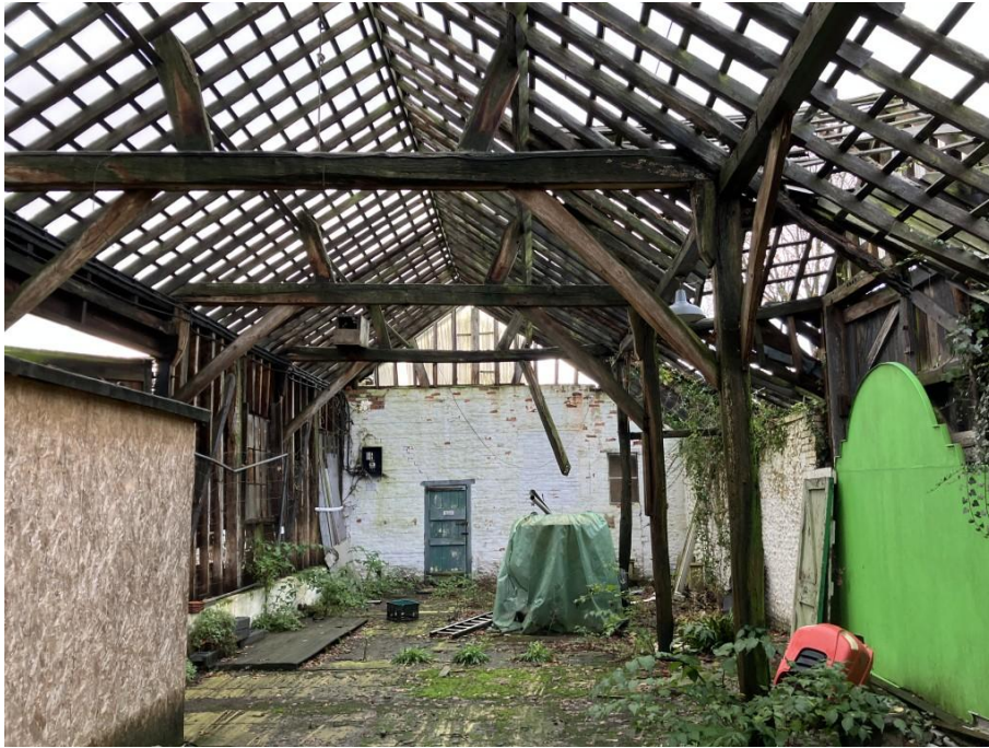
Photograph 25 – General view of barn structure looking to south. Note detached diagonal brace.
