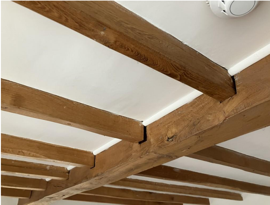
Photograph 13 – Open joints in timber indicates shallow connection of cosmetic joists.
