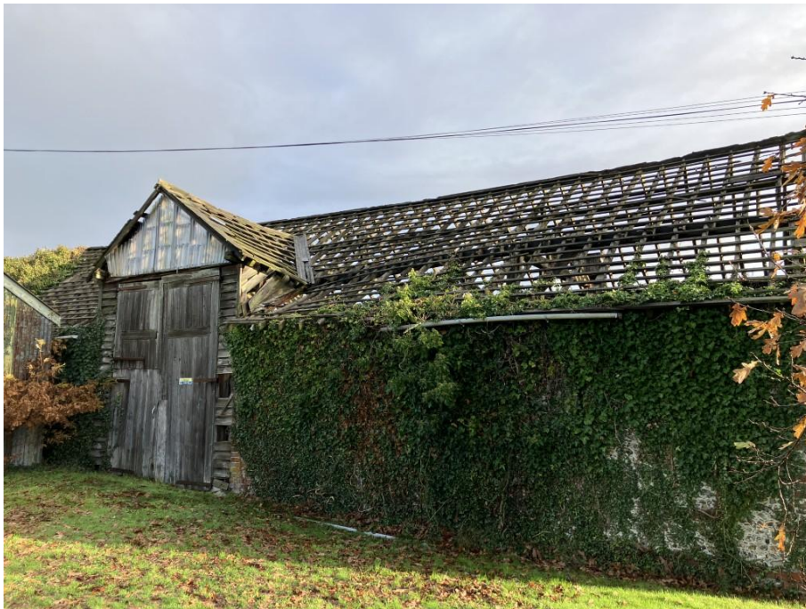
Photograph 26 – West elevation of barn. Note ivy coloured flint wall, degraded lower roof pitch and intersecting gable over western door.
