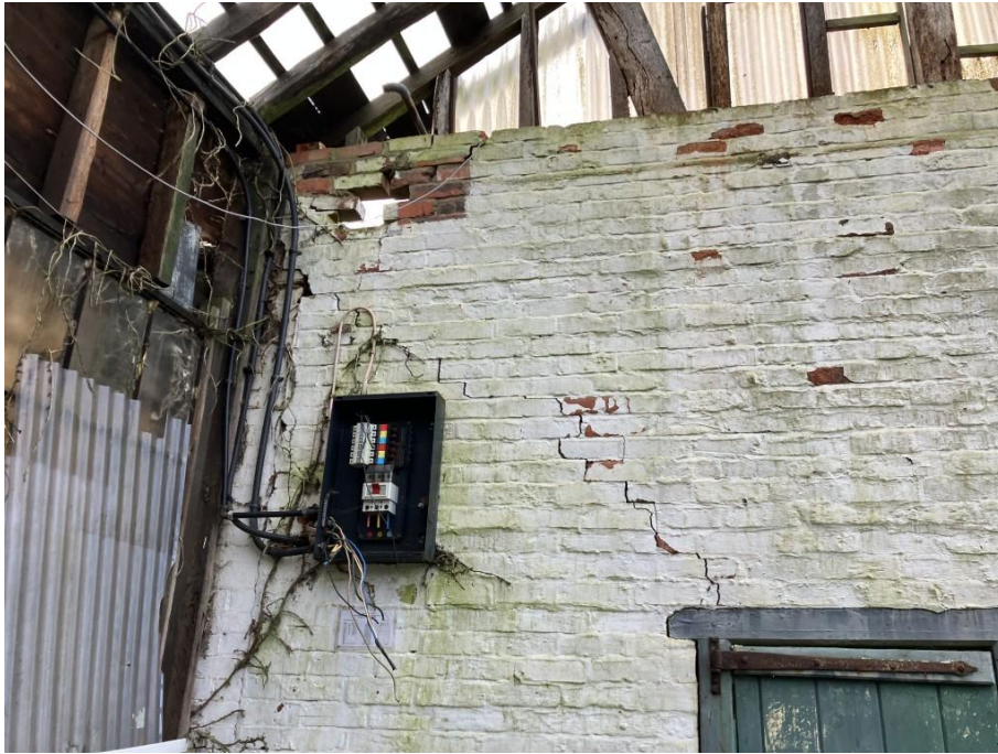
Photograph 29 – Cracking of brickwork infill wall to south elevation.
