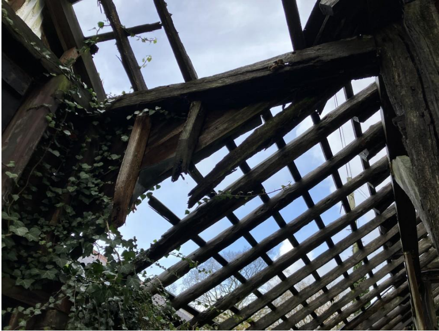
Photograph 35 – Severe decay and missing elements to cheek of intersecting gable.
