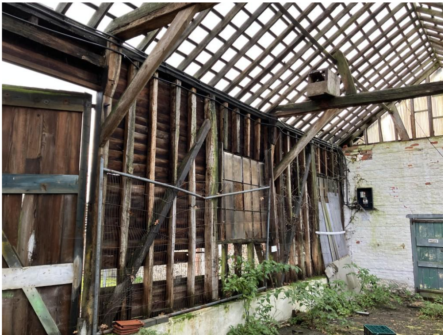
Photograph 32 – Large window openings former in east elevation without adequate timber framing. East elevation displaced by failure of timber structure shown in Photograph 34.
