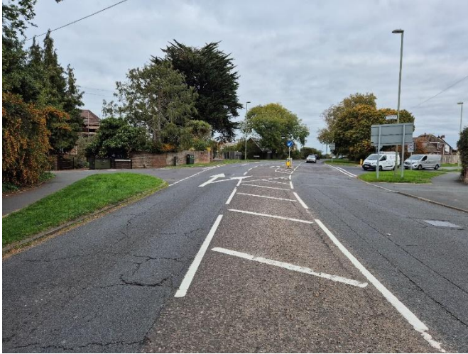
Photograph 79: Existing condition on Hulbert Road (B2150) (looking north heading towards Park Lane junction on right)
