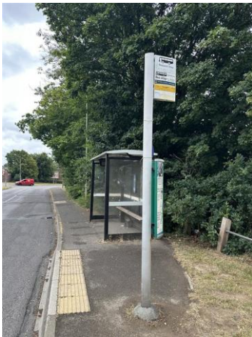
Photograph 26: Footway and bus stop condition on Calshot Road (Southern edge of carriageway)
