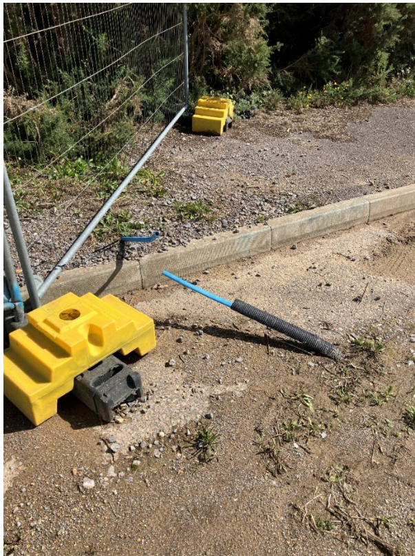
Figure 4: Historic / unfinished service runs at plot entrance
