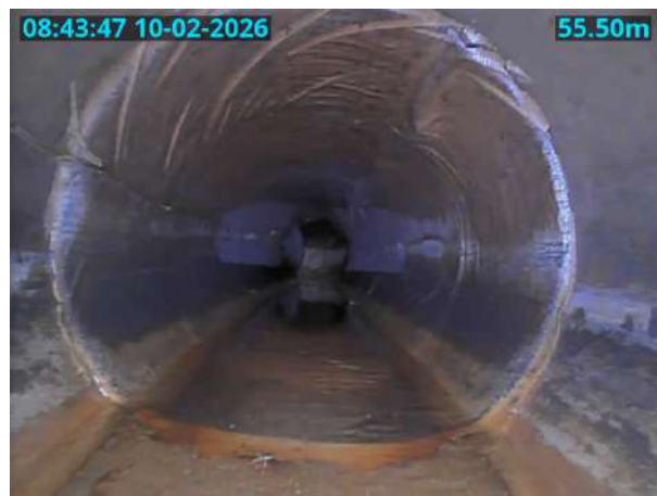
MH17X_D_10022026_0844_038.jpg, 00:05:36, 55.50 m Point repair, localised lining from 12 o'clock to 12 o'clock
