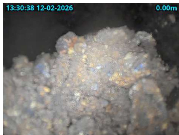
74AX_78c8c9e3-c7b2-4bf7-9723-678fc35ca4e8_20260223_143922_303.jpg, 00:00:17, 0.00 m Settled deposits, fine, 35% cross-sectional area loss
