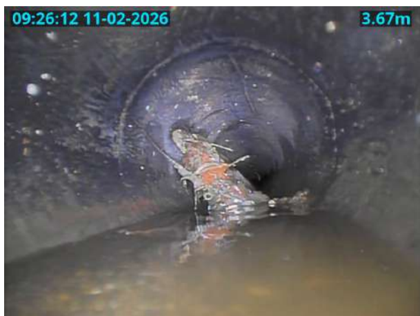
MH39X_D_11022026_0927_111.jpg, 00:00:35, 3.67 m Settled deposits, other, 40% cross-sectional area loss, Rubble / twiggs, Pushing
