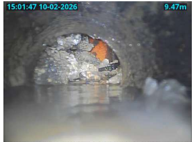
37BX_U_10022026_1501_068.jpg, 00:01:13, 9.47 m Collapsed drain or sewer, 70% cross-sectional area loss
