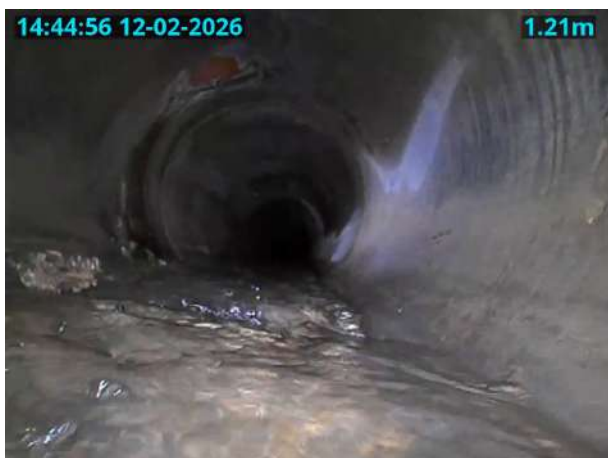
MH78X_39fa71cf-9ab2-4099-a4e1-105265ceb767_20260223_154432_527.jpg, 00:00:11, 0.00 m Settled deposits, coarse, 10% cross-sectional area loss, start
