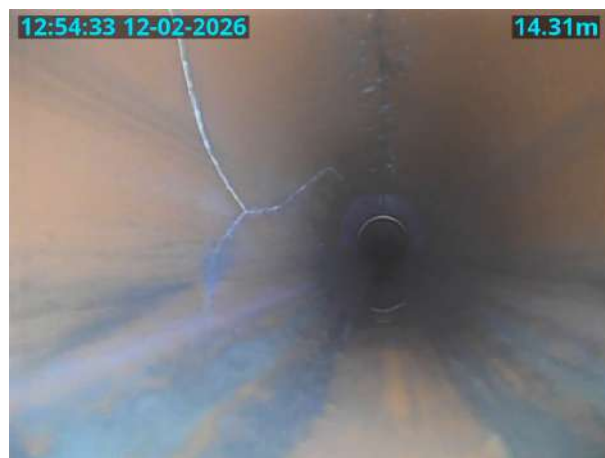
MH72X_5f7bf511-1f5d-40f5-87d9-1c871739e7cf_20260223_141551_135.jpg, 00:01:25, 14.31 m Crack, longitudinal at 9 o'clock
