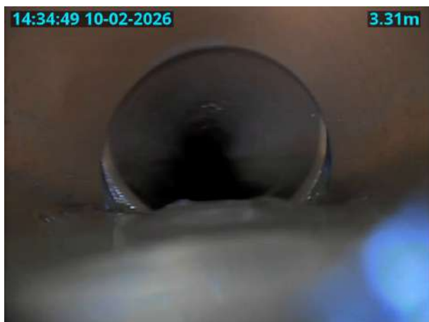
36AX_U_10022026_1435_063.jpg, 00:00:17, 3.31 m Joint displaced, medium
