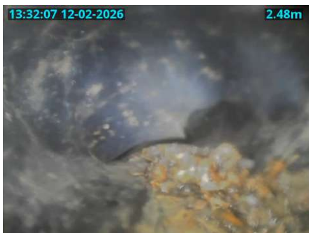
74CX_bd552570-be25-4d06-bce7-7bfd50653d20_20260223_150247_979.jpg, 00:00:21, 2.48 m Deformed sewer or drain, 80%, SQUASHED PIPE
