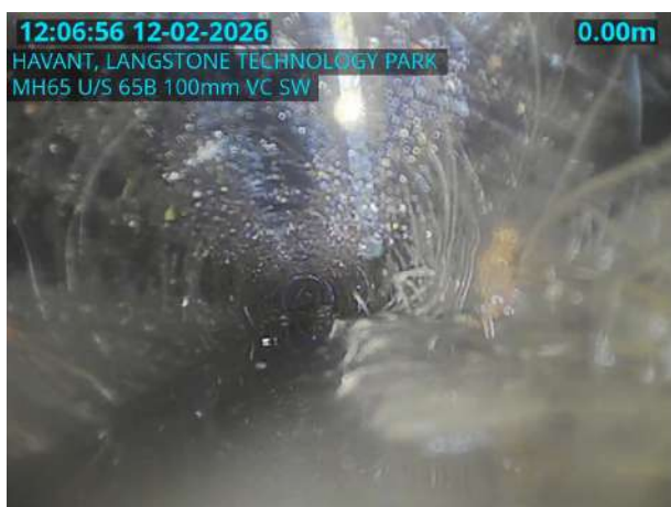
65BX_cc464784-8f3f-48e0-b571-1108eed4f1f5_20260223_134846_758.jpg, 00:00:01, 0.00 m Settled deposits, fine, 20% cross-sectional area loss, start
