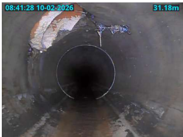
MH17X_D_10022026_0844_037.jpg, 00:03:17, 31.18 m Connection defective, connecting pipe is intruding at 10 o'clock, 100mm dia, intrusion: 10%
