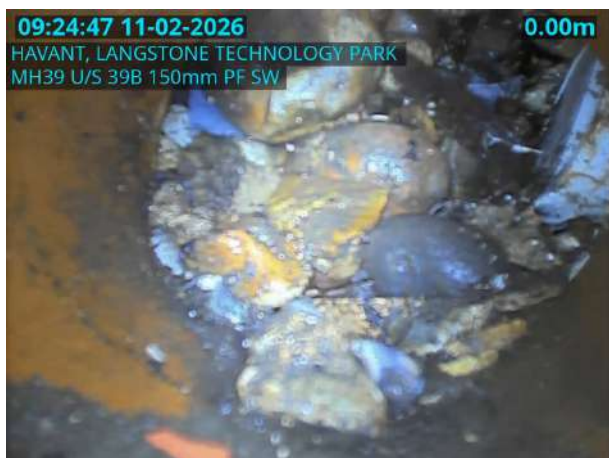
39BX_U_11022026_0924_110.jpg, 00:00:03, 0.00 m Settled deposits, coarse, 100% cross-sectional area loss
