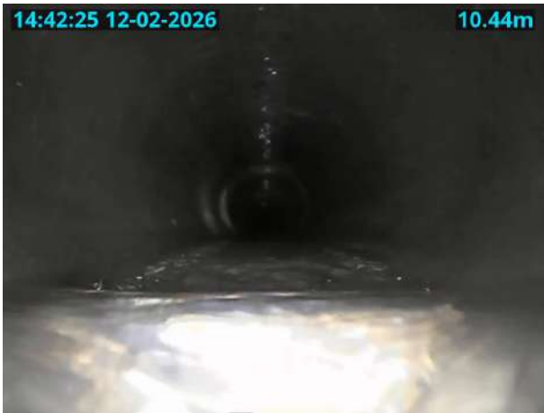
MH76X_fd8ccc54-4fd8-42fe-8163-c02797994899_20260223_154041_077.jpg, 00:01:12, 10.44 m Settled deposits, coarse, 15% cross-sectional area loss
