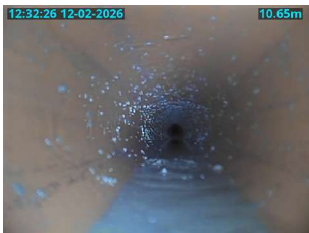
67BX_d06e8542-cadb-4520-8807-97cf7d1b7d27_20260223_140759_394.jpg, 00:01:13, 10.65 m Settled deposits, fine, 5% cross-sectional area loss
