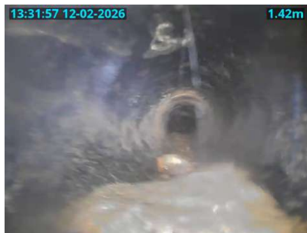
74CX_bf3e348a-2beb-416e-b662-05e4b08a42e7_20260223_150208_702.jpg, 00:00:11, 1.42 m Settled deposits, coarse, 10% cross-sectional area loss
