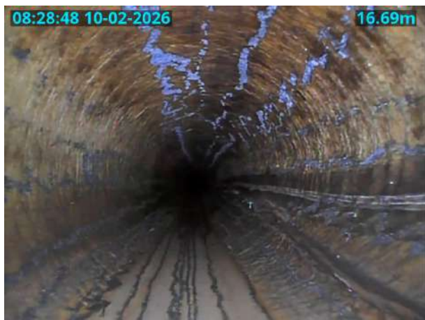
MH19X_U_10022026_0831_100.jpg, 00:02:34, 16.69 m Defective lining, wrinkled (longitudinal) at 5 o'clock
