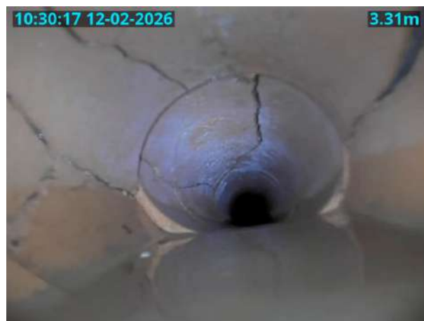
MH53X_8e46ed57-625e-4987-9bd9-86e2f09b960e_20260223_133332_225.jpg, 00:00:19, 3.31 m Joint displaced, large
