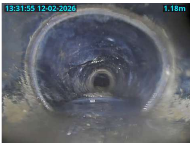
74CX_0a3ddfd2-5c01-43a4-95a6-6f60dc623085_20260223_150152_097.jpg, 00:00:09, 1.18 m Deformed sewer or drain, 10%
