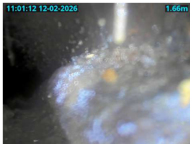
MH56X_04ceadd2-c3ea-4a61-a940-9907a48c0365_20260223_134058_224.jpg, 00:00:18, 1.66 m Settled deposits, hard or compacted, 30% cross-sectional area loss, change
