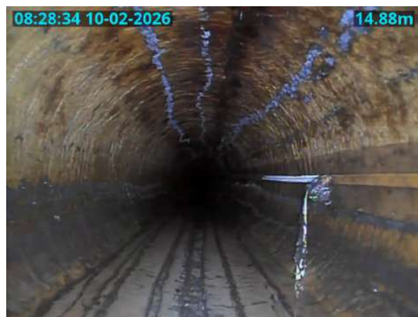
MH19X_U_10022026_0831_099.jpg, 00:02:20, 14.88 m Defective lining, separated seam cover at 4 o'clock
