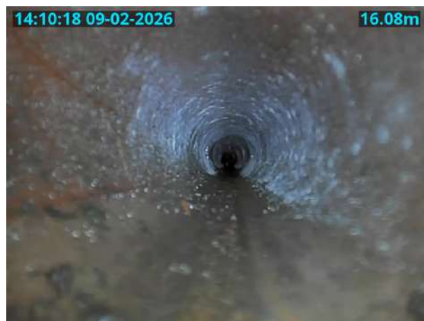
12AX_U_09022026_1411_027.jpg, 00:01:41, 16.08 m Fracture, longitudinal at 10 o'clock
