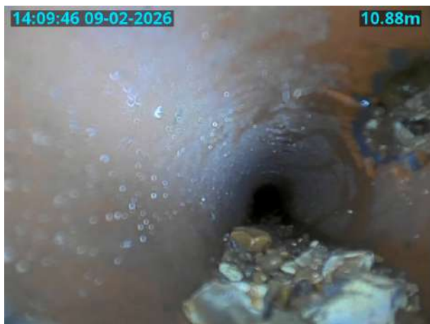
12AX_U_09022026_1411_024.jpg, 00:01:09, 10.88 m Hole in drain or sewer from 1 o'clock to 3 o'clock
