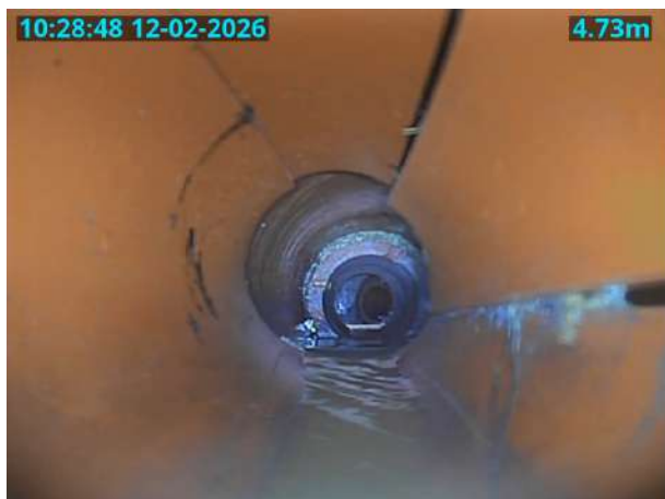
MH54X_98b183b6-1514-4a1d-be7d-1fe61282fcc6_20260223_125738_012.jpg, 00:01:17, 4.73 m Defective repair, other from 12 o'clock to 12 o'clock, PIPE JOINING DEFECTIVE
