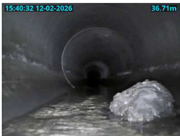
MH80X_ea6cf17c-1c75-45b5-8a8a-b7ace45a023d_20260223_155813_822.jpg, 00:03:05, 36.71 m Settled deposits, coarse, 15% cross-sectional area loss, STONE
