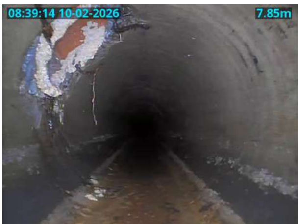
MH17X_D_10022026_0844_035.jpg, 00:01:03, 7.85 m Connection defective, connecting pipe is intruding at 10 o'clock, 100mm dia, intrusion: 10%
