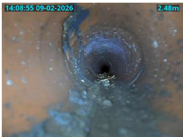
12AX_U_09022026_1411_022.jpg, 00:00:18, 2.48 m Hole in drain or sewer from 9 o'clock to 11 o'clock
