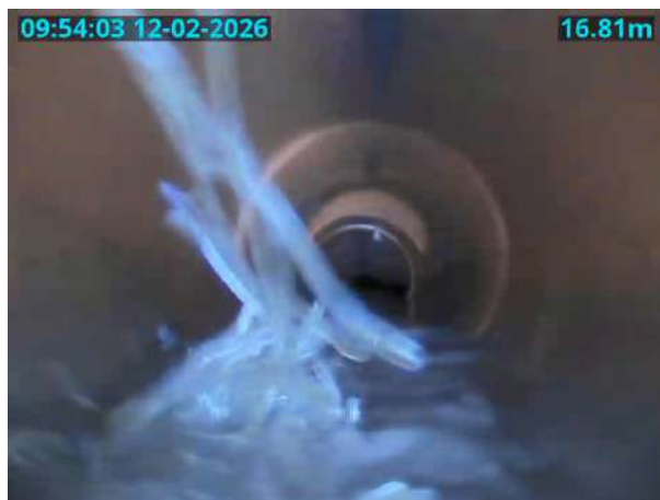
MH50X_c4d21d95-e803-416a-bae8-30b0d6476027_20260223_123447_718.jpg, 00:01:57, 16.81 m Roots, mass, 10% cross-sectional area loss
