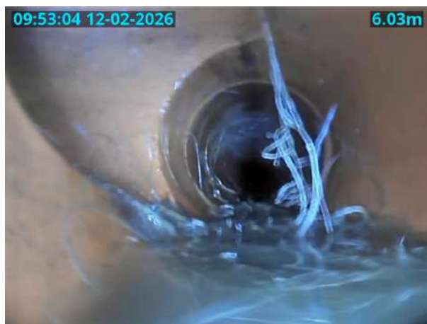
MH50X_4b2c89ca-b867-4f42-ba8d-87102b712706_20260223_123235_731.jpg, 00:00:59, 6.03 m Junction at 10 o'clock, 100mm dia
