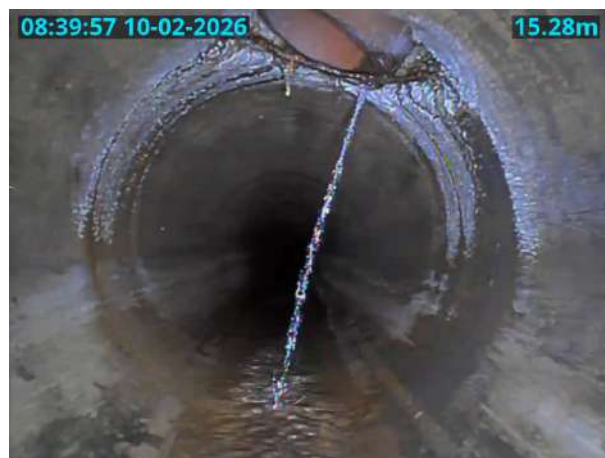
MH17X_D_10022026_0844_036.jpg, 00:01:46, 15.28 m Connection defective, connecting pipe is intruding at 1 o'clock, 100mm dia, intrusion: 10%, Live
