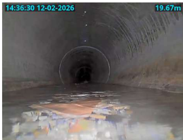
MH25X_8dbbfdc4-b1cd-42b9-8592-dfeec2f6ace1_20260223_153441_311.jpg, 00:01:36, 23.93 m Settled deposits, coarse, 20% cross-sectional area loss, change, LARGE STONE
