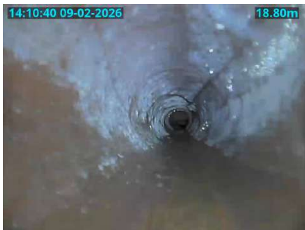
12AX_U_09022026_1411_028.jpg, 00:02:03, 18.80 m Fracture, longitudinal at 10 o'clock
