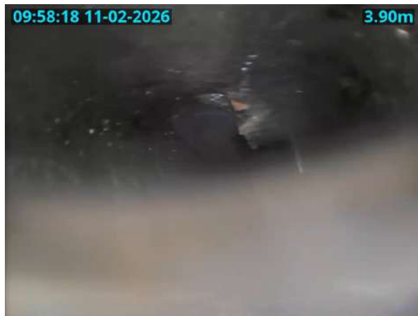
MH41X_D_11022026_0958_113.jpg, 00:00:24, 3.90 m Hole in drain or sewer at 12 o'clock
