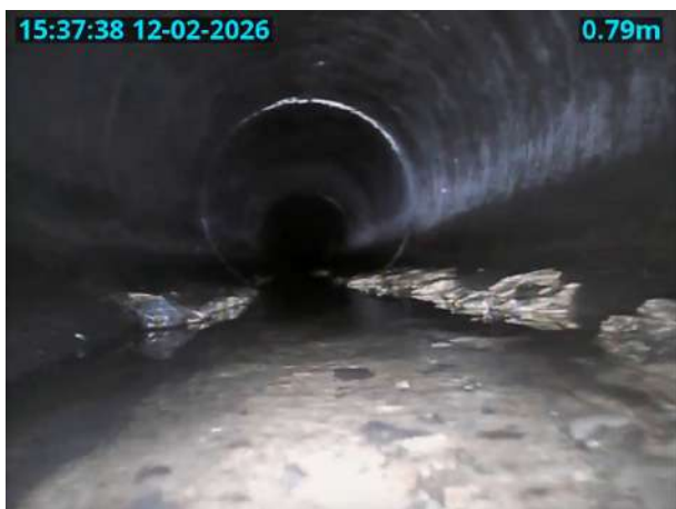
MH80X_5b86b685-05e6-4278-9c48-a11944ee3266_20260223_155607_481.jpg, 00:00:11, 0.00 m Settled deposits, fine, 5% cross-sectional area loss, start
