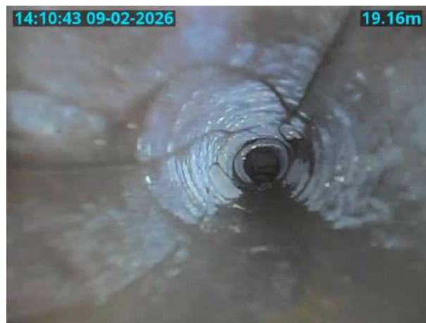
12AX_U_09022026_1411_029.jpg, 00:02:06, 19.16 m Fractures, multiple from 12 o'clock to 12 o'clock
