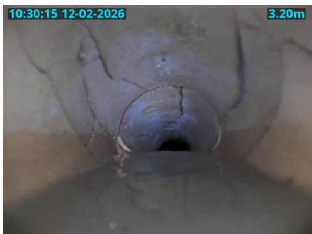
MH53X_5374aaaf-4b5d-4cd3-a655-1d9ca2669697_20260223_133317_973.jpg, 00:00:17, 3.20 m Fractures, multiple from 12 o'clock to 12 o'clock
