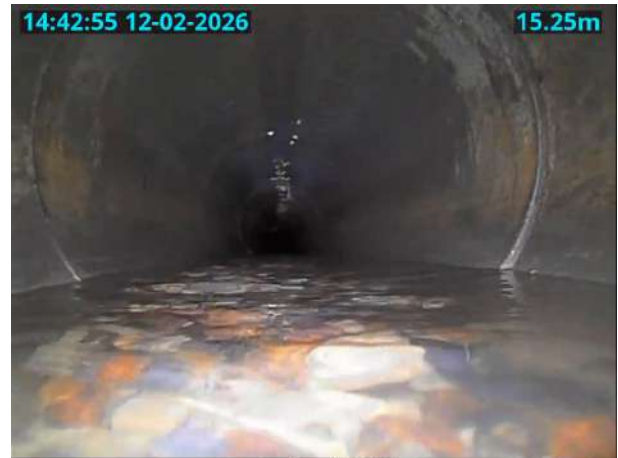
MH76X_52cbf0c5-166a-4477-96cd-043014f41dee_20260223_154115_591.jpg, 00:01:42, 15.25 m Settled deposits, coarse, 10% cross-sectional area loss, start
