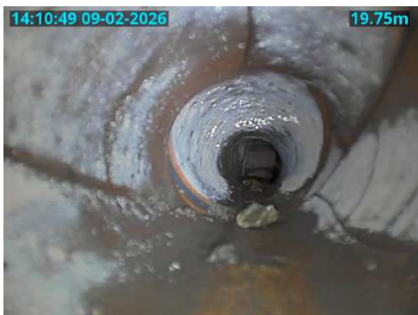
12AX_U_09022026_1411_030.jpg, 00:02:12, 19.75 m Broken pipe from 2 o'clock to 8 o'clock
