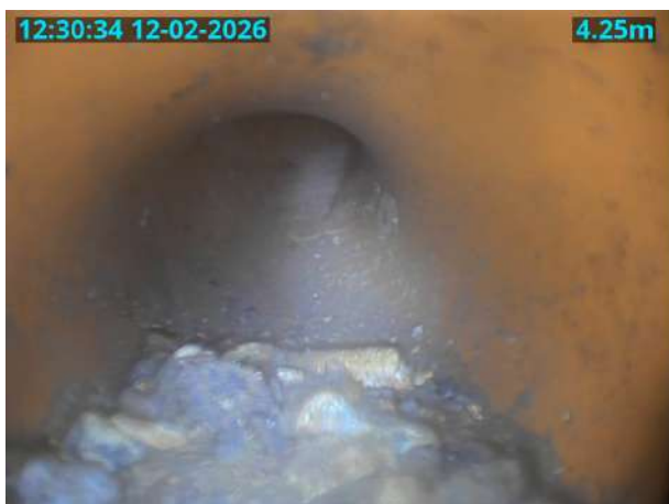
67AX_e712470a-26e3-4134-b2d9-cdc196dac5e0_20260223_140250_670.jpg, 00:00:29, 4.25 m Settled deposits, coarse, 10% cross-sectional area loss, finish
