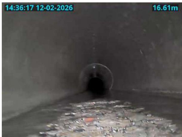
MH25X_4aee4e54-6064-4f62-9aa3-2db974a143af_20260223_153356_347.jpg, 00:01:23, 16.61 m Settled deposits, fine, 10% cross-sectional area loss, start
