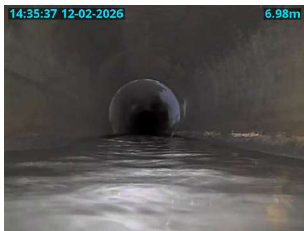
MH25X_69069a43-4ba9-4455-8549-41131022f3ba_20260223_153256_801.jpg, 00:00:43, 6.98 m Settled deposits, coarse, 10% cross-sectional area loss, finish
