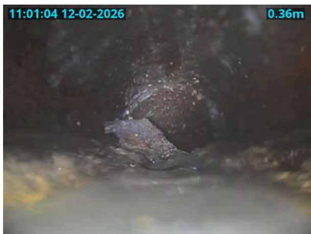
MH56X_f6baea80-03cf-48b7-8a11-8c1329f72436_20260223_134022_818.jpg, 00:00:10, 0.36 m Settled deposits, hard or compacted, 20% cross-sectional area loss, start
