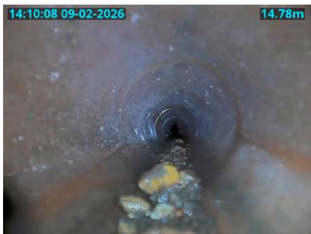
12AX_U_09022026_1411_026.jpg, 00:01:31, 14.78 m Fracture, circumferential from 7 o'clock to 5 o'clock
