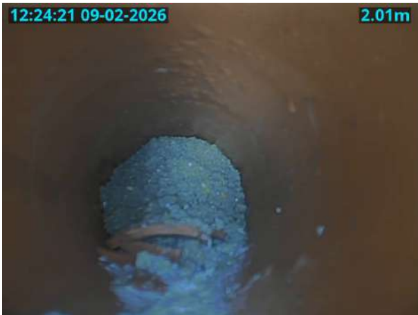
11AX_U_09022026_1224_013.jpg, 00:00:17, 2.01 m Collapsed drain or sewer, 100% cross-sectional area loss
