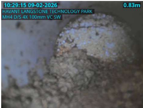
MH4X_D_09022026_1029_088.jpg, 00:00:09, 0.83 m General remark, Line capped
