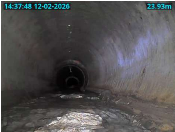
MH25X_9838f1f9-094c-47cc-9e38-5bdfc7f75e6e_20260223_1 53549_810.jpg, 00:01:36, 23.93 m Settled deposits, coarse, 20% cross-sectional area loss, change, LARGE STONE
