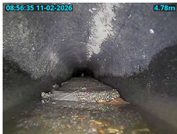
MH38X_D_11022026_0856_073.jpg, 00:01:01, 4.78 m Other obstacles, other object in invert from 4 o'clock to 8 o'clock, 40% cross-sectional area loss, Wood
