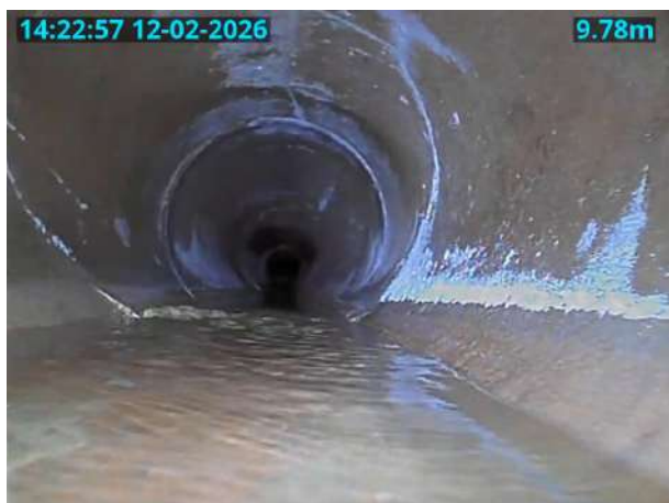
MH77X_862cbb0e-d4d0-42e5-bf4e-b5bfd886099d_20260223_152521_276.jpg, 00:01:46, 9.78 m Cracks, multiple from 12 o'clock to 12 o'clock
