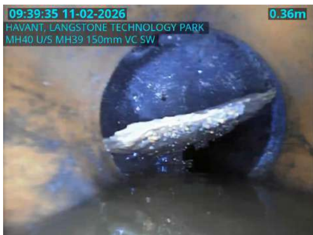
MH39X_U_11022026_0939_079.jpg, 00:00:03, 0.36 m Settled deposits, coarse, 40% cross-sectional area loss
