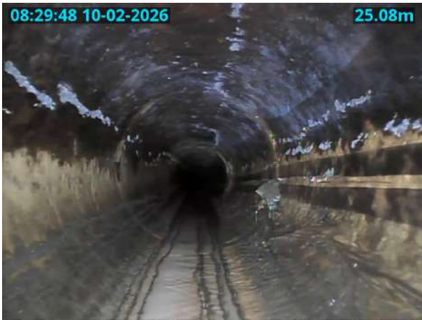
MH19X_U_10022026_0831_102.jpg, 00:03:34, 25.08 m Defective lining, wrinkled (longitudinal) at 4 o'clock
