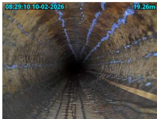
MH19X_U_10022026_0831_101.jpg, 00:02:55, 19.26 m Defective lining, separated seam cover at 4 o'clock
