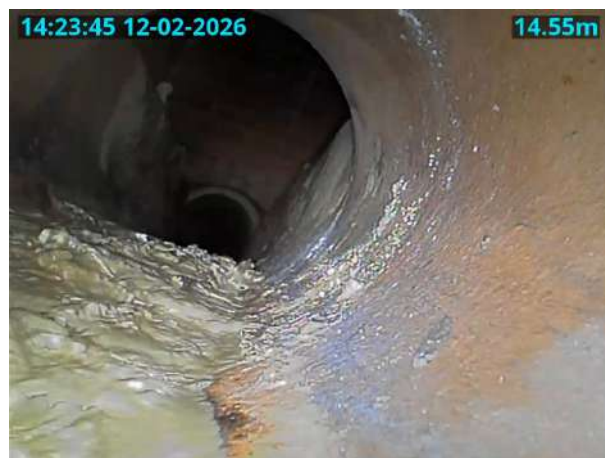
MH77X_8bdec740-7ab5-4919-9999-e70e024a8245_20260223_152625_484.jpg, 00:02:34, 14.55 m Settled deposits, fine, 15% cross-sectional area loss, DEBRIS BUILD UP IN MANHOLE
