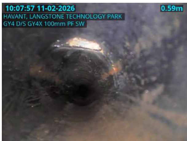
GY4X_D_11022026_1009_083.jpg, 00:00:03, 0.59 m Hole in drain or sewer at 12 o'clock
