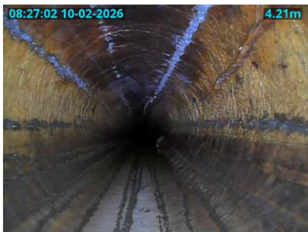
MH19X_U_10022026_0831_098.jpg, 00:00:48, 4.21 m Defective lining, wrinkled (longitudinal) at 2 o'clock
