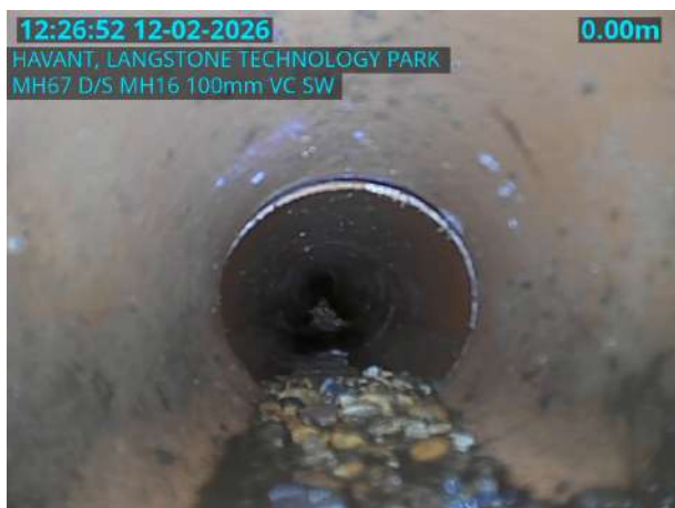
MH67X_e6423dbc-9058-4b13-915d-2083dd1ee47e_20260223_135555_032.jpg, 00:00:01, 0.00 m Settled deposits, coarse, 10% cross-sectional area loss, start, STONES AND SILT
