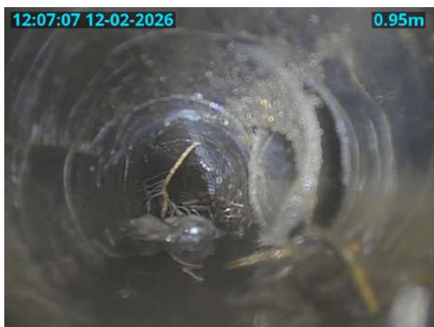
65BX_c4d8bf0a-1aea-42f5-ad13-460709ea9ac4_20260223_134947_099.jpg, 00:00:12, 0.95 m Connection other than junction at 3 o'clock, 100mm dia
