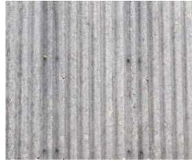
Existing asbestos cement sheeting
