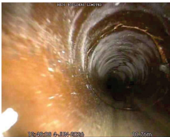
3, 00:01:22, 10.76 m Circumferential crack from 9 o'clock to 3 o'clock, Cracked pipe.
