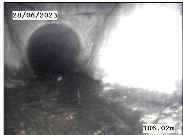
SW02X_11044567-ae19-4cef-a36c-147163cb4393_20230628_092714_874.jpg, 00:05:21, 106.02 m Finish node, manhole, reference: SW02
