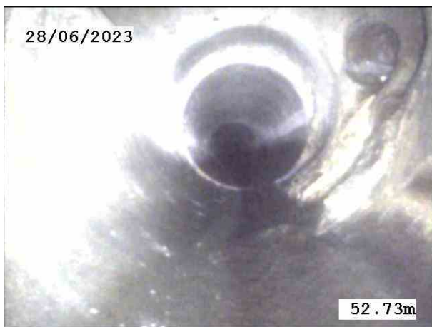
SW03X_a412e238-8a50-4a95-9ffe-6d634b25808c_20230628_095743_568.jpg, 00:03:50, 52.73 m Finish node, manhole, reference: SW03, Buried unable to locate
