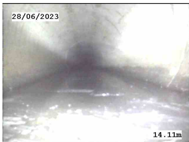
SW01X_fba8b68b-b436-4577-8445-55d7af249511_20230628_091003_638.jpg, 00:01:35, 14.11 m Water level, 10% of the vertical dimension
