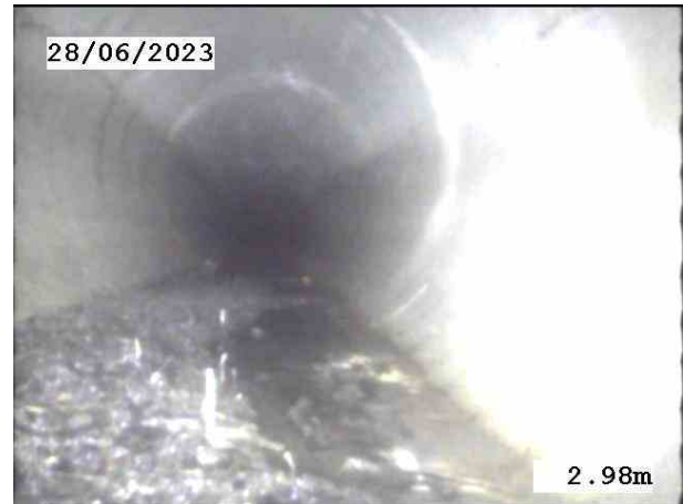
SW02X_3f214bcc-a7be-46a5-b6e9-504499828465_20230628_092208_139.jpg, 00:00:28, 2.98 m Settled deposits, hard or compacted, 5% cross-sectional area loss
