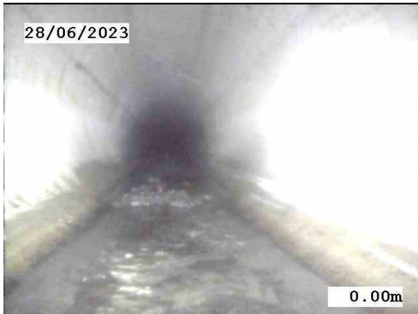
SW02X_ca9b5fb1-3733-43b7-b3af-b8b7884a0209_20230628_092127_673.jpg, 00:00:01, 0.00 m Start node, manhole, reference: SW01
