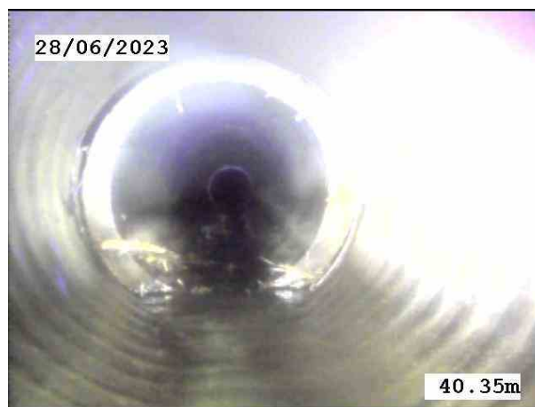
SW04X_114fe8d6-cb27-4c11-bd70-7e086f1c94d1_20230628_103302_372.jpg, 00:03:34, 40.35 m Joint displaced, large
