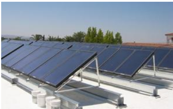
Figure 7 – Frame mounted panels on flat roof
