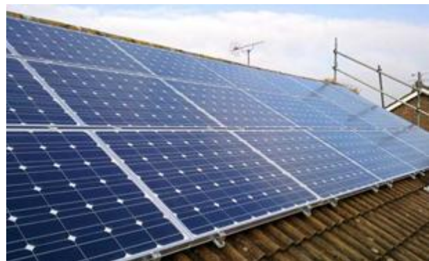
Figure 8 - Roof mounted panels
