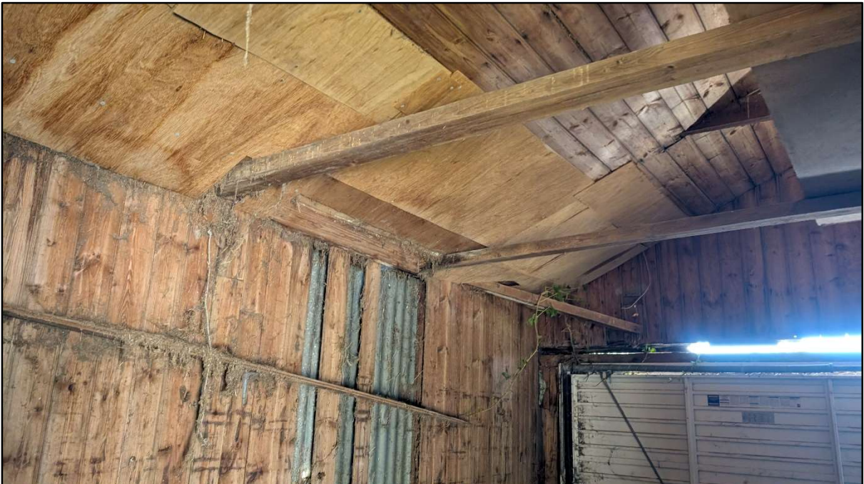
Photo 10 – Nesting material visible between the corrugated metal walls and wooden sarking.
