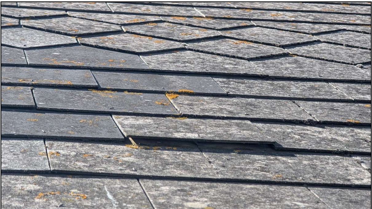
Photo 4 – View of a lifted tile on the roof of B1.
