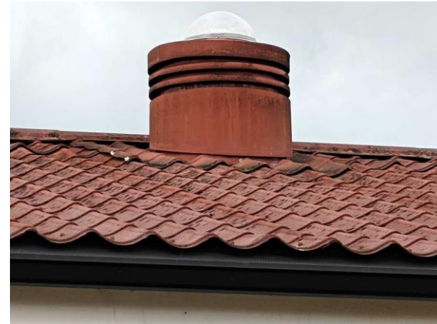
Western aspect of the roof of building B1 showing gaps
