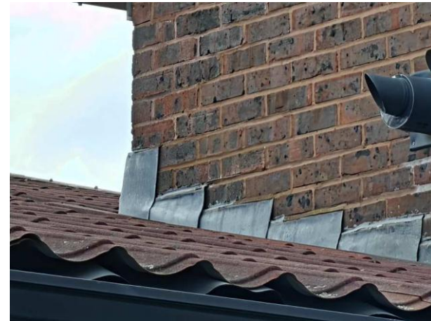
Western aspect of building B1 showing gaps underneath areas of raised lead flashing
