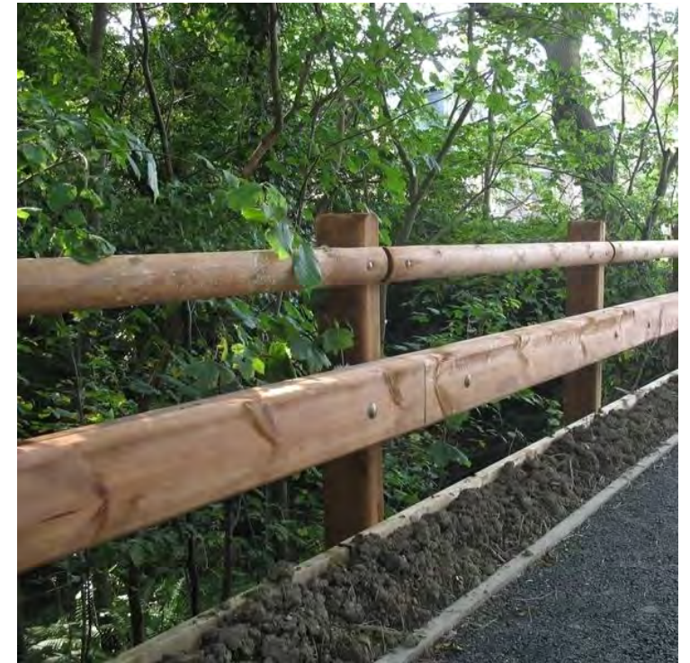
Timber vehicle restraint fencing
