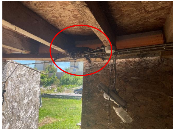
Photo 8 – Old bird nest in building 4.
