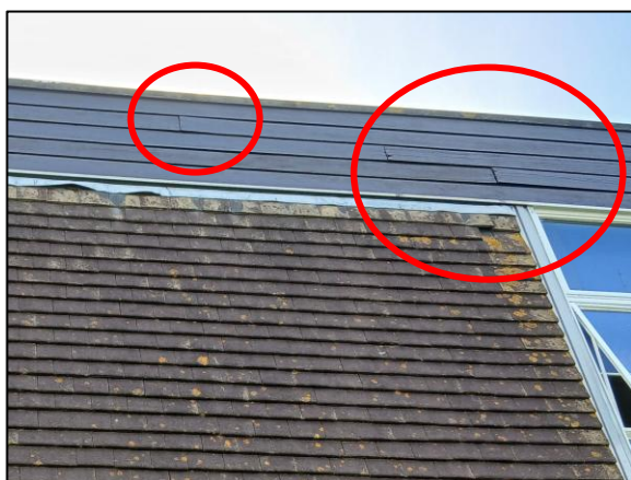
Photo 3 Western elevation – gaps in timber cladding
