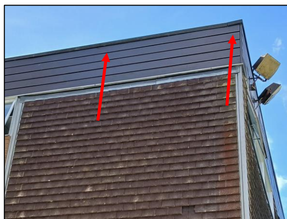
Photo 4 Southern elevation – Gaps under overlap at top of external wall
