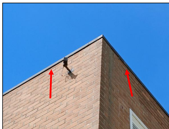
Photo 8 Southern elevation – gaps under overlap at top of exterior walls
