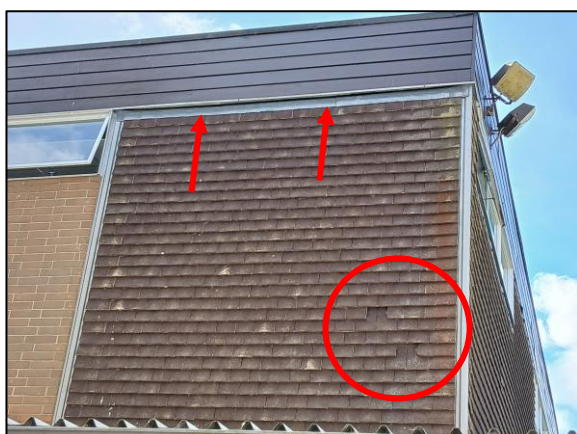
Photo 5 Southern elevation – missing tiles (red circle), gap at top of lead flashing (red arrows)
