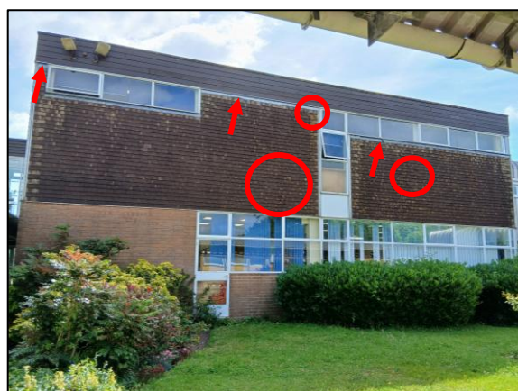
Photo 6 Western elevation – missing tiles (red circles) gaps around lead flashing (red arrows)
