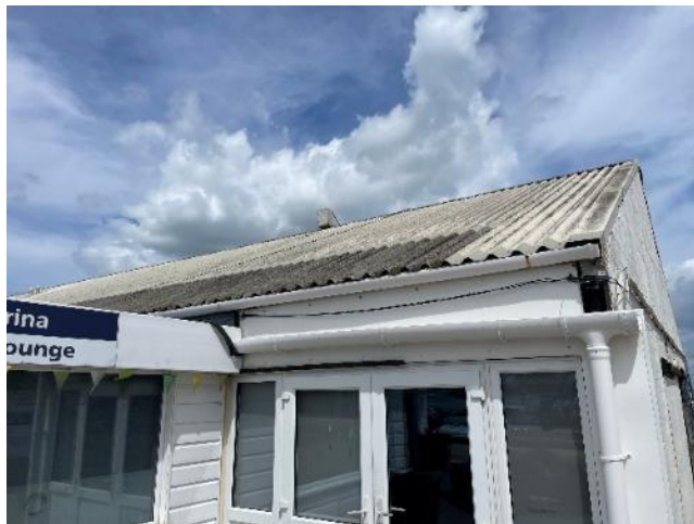
Eastern elevation showing gaps at the base of the roof
