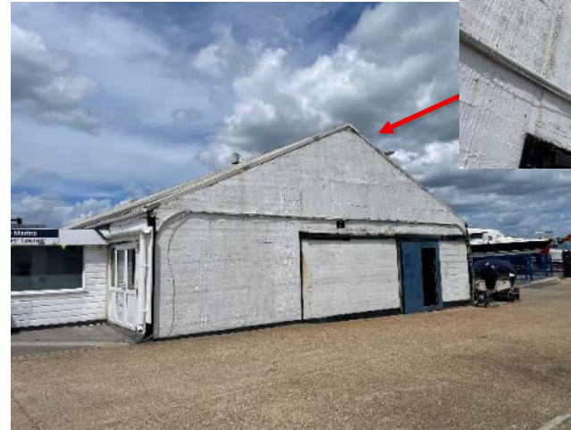
Southern elevation showing a gap between the gable end and roof overhang
