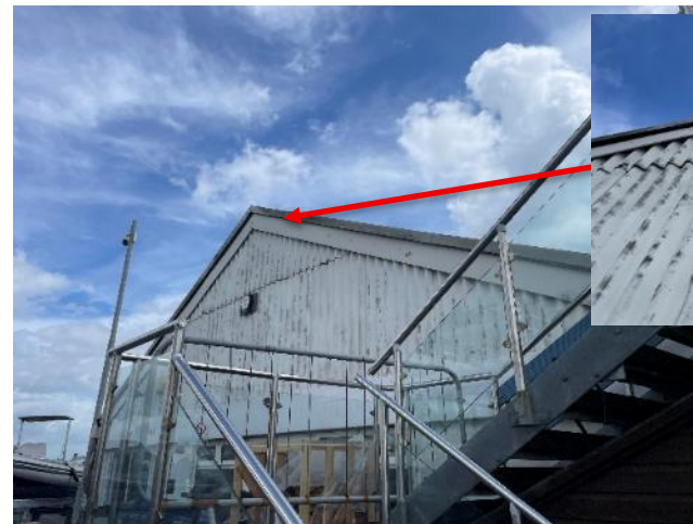
Northern elevation showing a gap between the gable end and roof overhang
