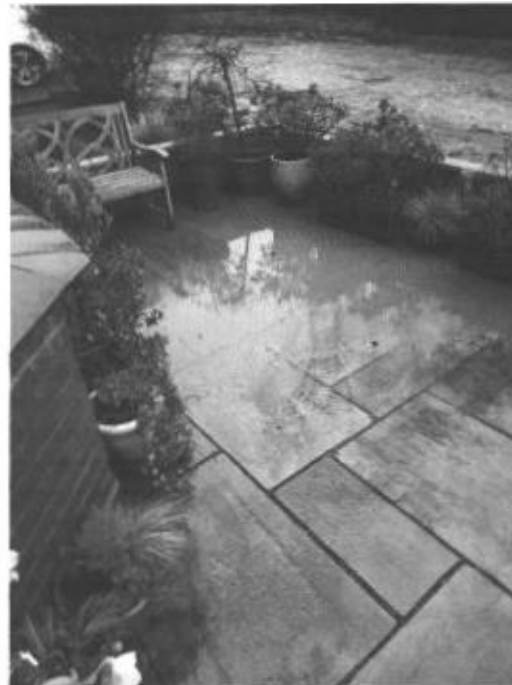
Photo 5: Standing water in my front garden at no.6
