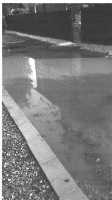
Photo 2: Flooding on The Dell access road
